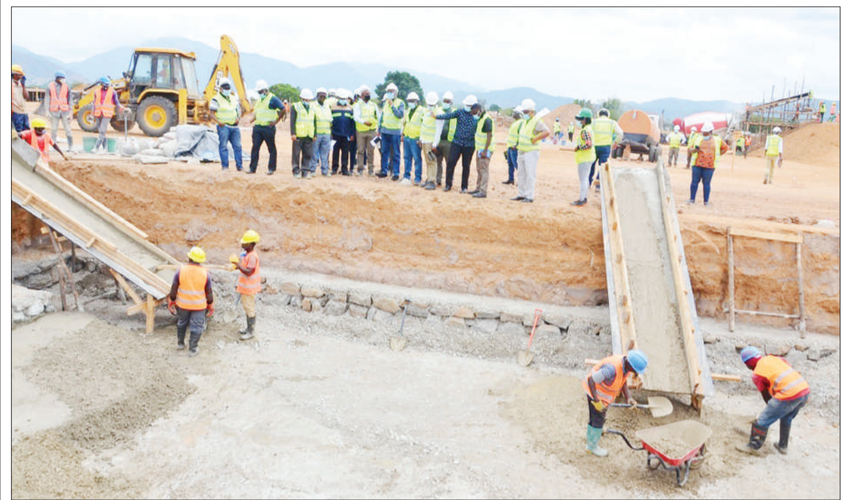
Members of the Rural Energy Agency board on a tour of an electric power station project at Ifakara in Morogoro Region yesterday. Photo: Guardian Correspondent
