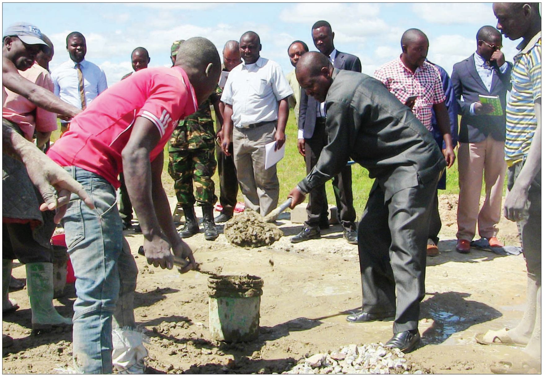
Rukwa Regional Commissioner Joachim Wangabo (C) participates on the ongoing construction of the Kalambo district hospital, during his official visit on Thursday. Photo: Guardian Correspondent
