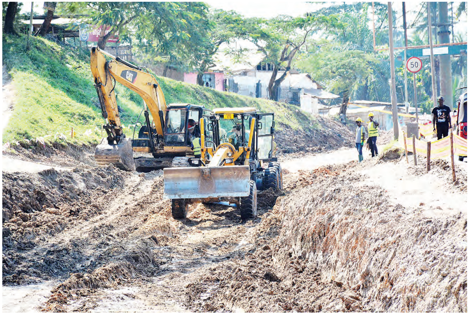
Major works along the Ubungo-Kimara Mwisho stretch of Dar es Salaam's Morogoro Road in progress yesterday. Photo: Correspondent Miraji Msala
