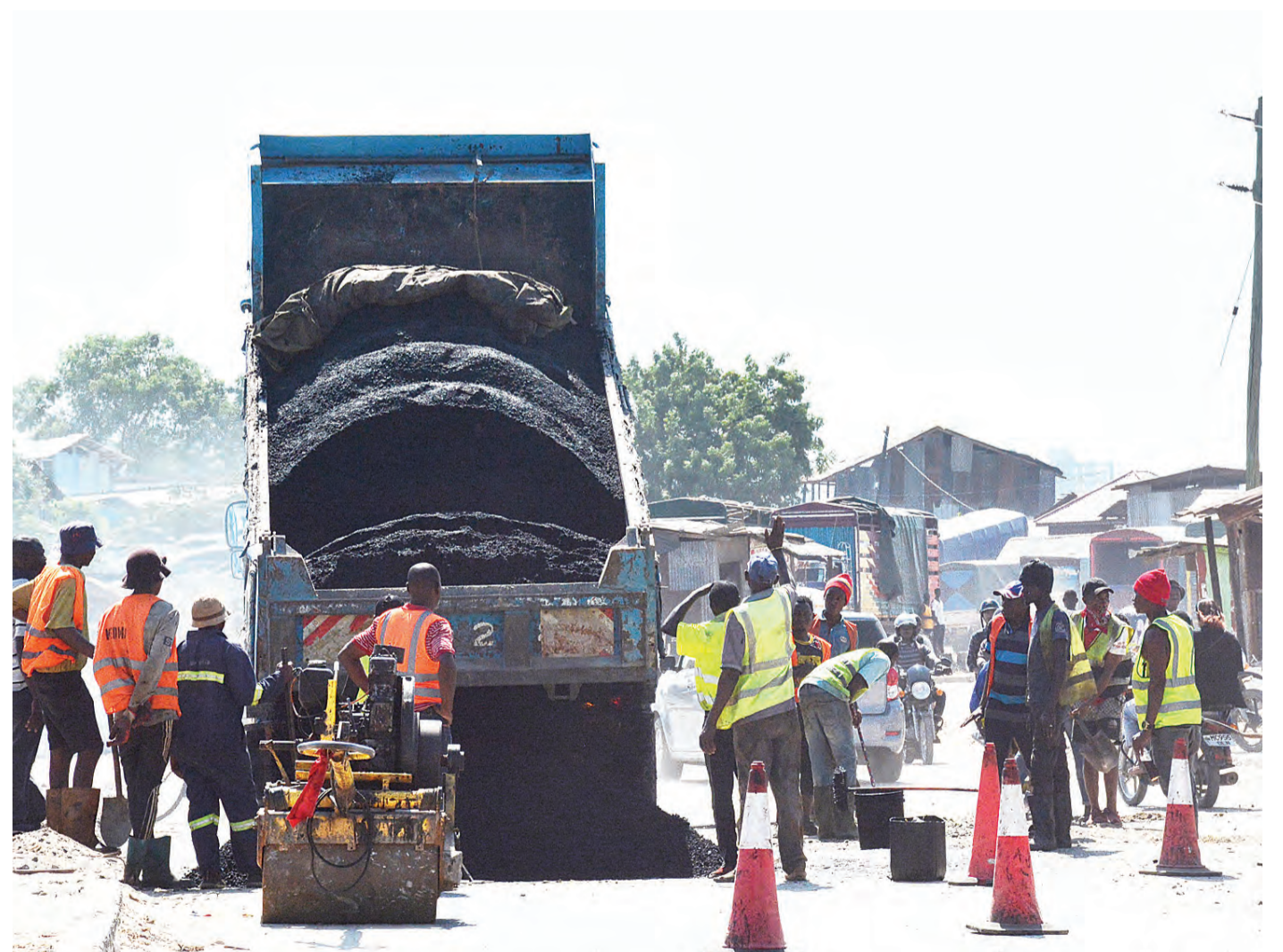
Rehabilitation of a section of a road at Kigogo-Sambusa in Ilala municipality, Dar es Salaam, well under way yesterday. Photo: Correspondent Miraji Msala
