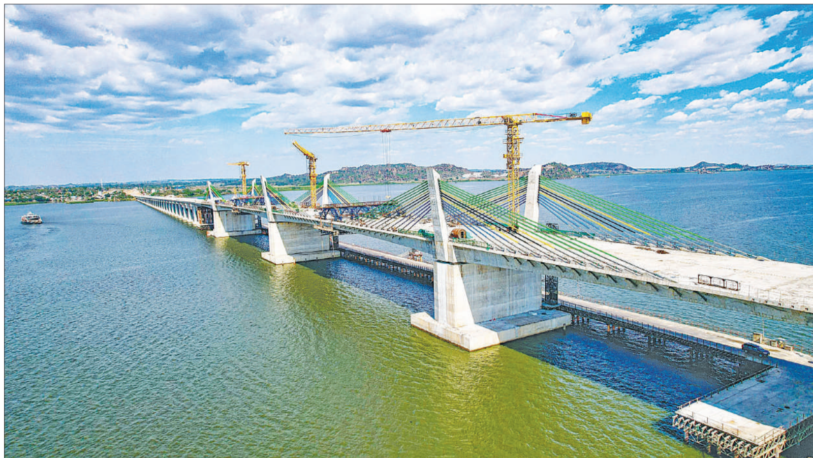
Aerial view of the 3-km Kigongo-Busisi J. P. Magufuli Bridge, which constitutes a section of the Usagara-Sengerema-Geita road across Lake Victoria waters and whose construction has reached the 93 per cent mark, as captured by the Works ministry on Sunday.
