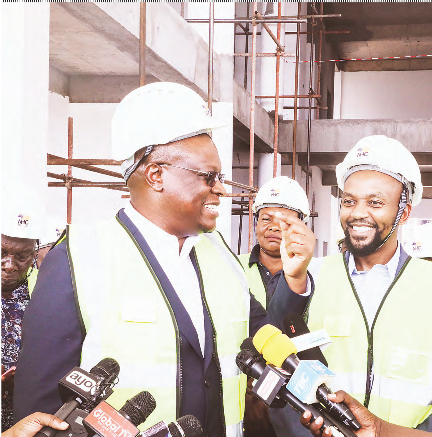
Information, Communications and Information Technology minister Nape Nnauye (in sunglasses) briefs journalists in Dodoma city yesterday shortly after making an assessment tour of progress in the construction of the ministry's office complex in the national capital's Mtumba suburb. Photo courtesy of Maelezo
