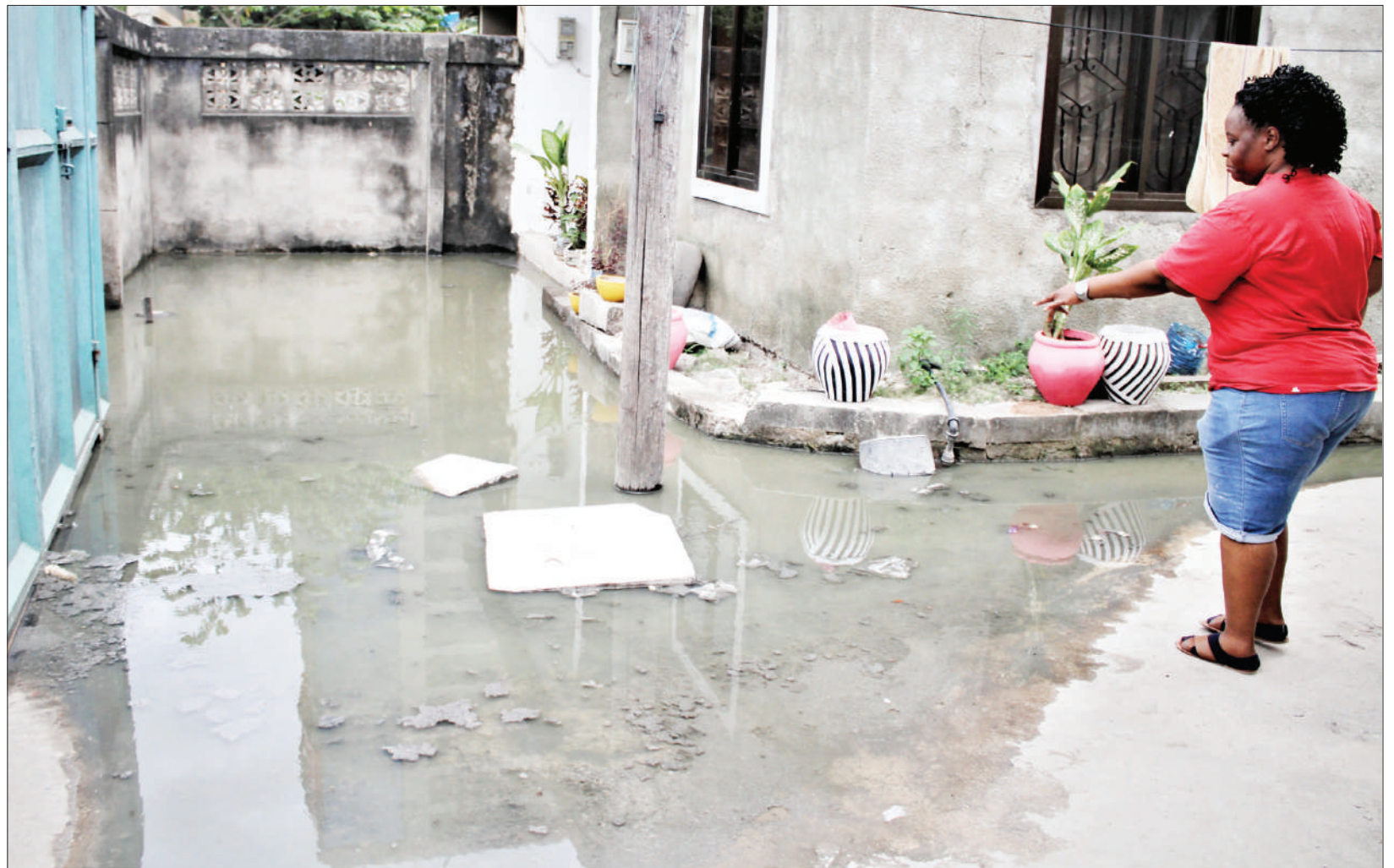
A Bwawani resident at Makumbusho area of Kijitonyama ward in Dar es Salaam, points at filthy and hazardous waste water surrounding one of the houses left in that state for four months now, on account of a flawed drainage situation, as captured yesterday. Photo: Guardian Correspondent
