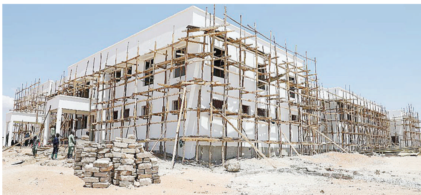
Construction work of Uhuru Hospital in Chamwino District is in progress. Photo courtesy of Airtel Tanzania.
