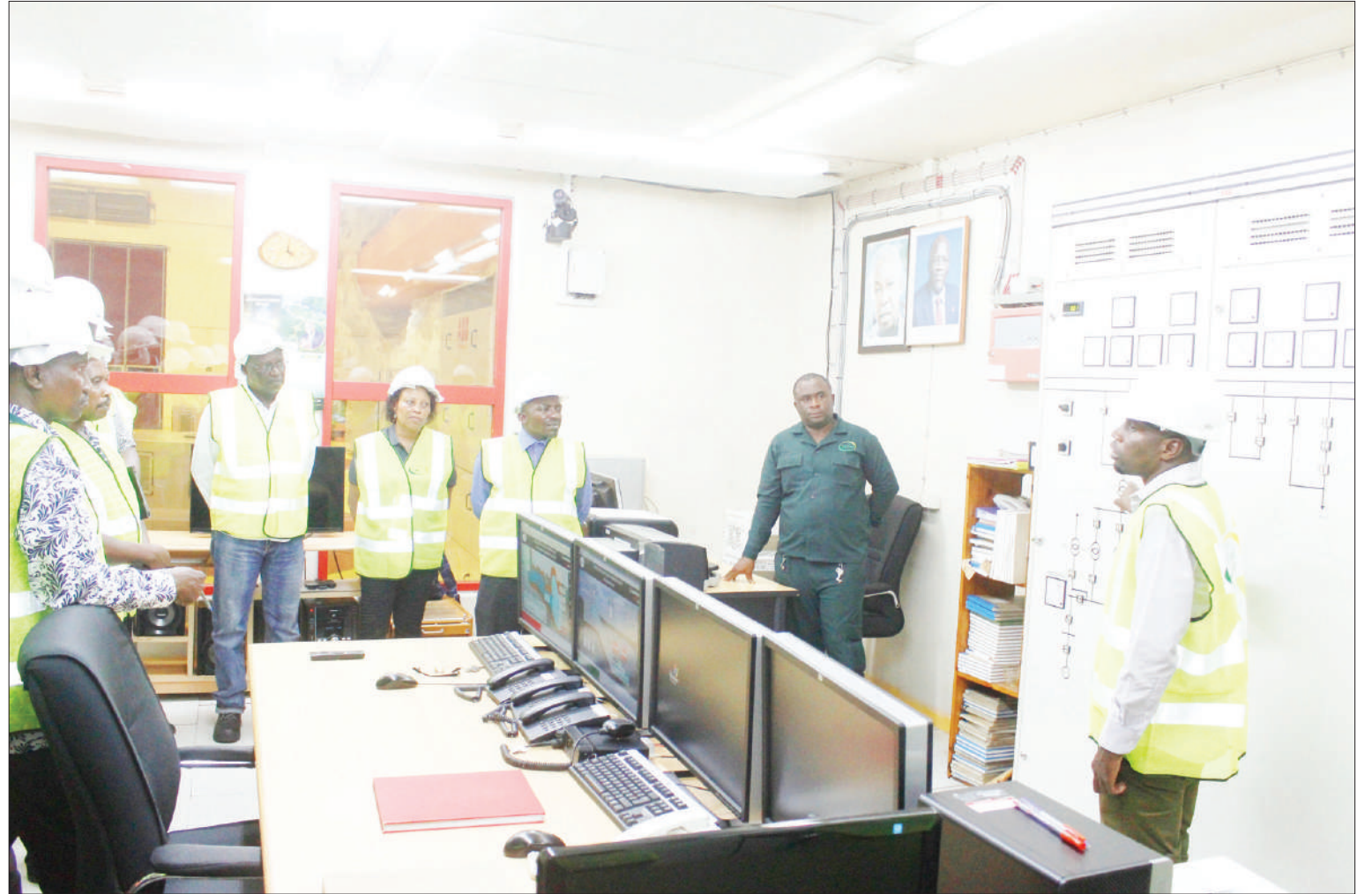
New Pangani Falls production engineer Dalali Lunyamila (R) briefs Tanzania Electric Supply Company (Tanesco) board members on operations at the Hale power generation plant in Korogwe District at the weekend. Photo: Correspondent Oscar Kasimiri
