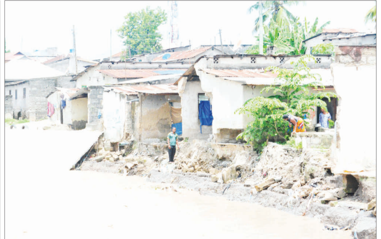
Houses in Dar es Salaam's Tandale kwa Mtogole suburb at serious risk of crumbling, what with the intermittent heavy rain the city is experiencing and the fact that they are already in poor shape. This scene was captured on Monday. Photo: Correspondent Miraji Msala
