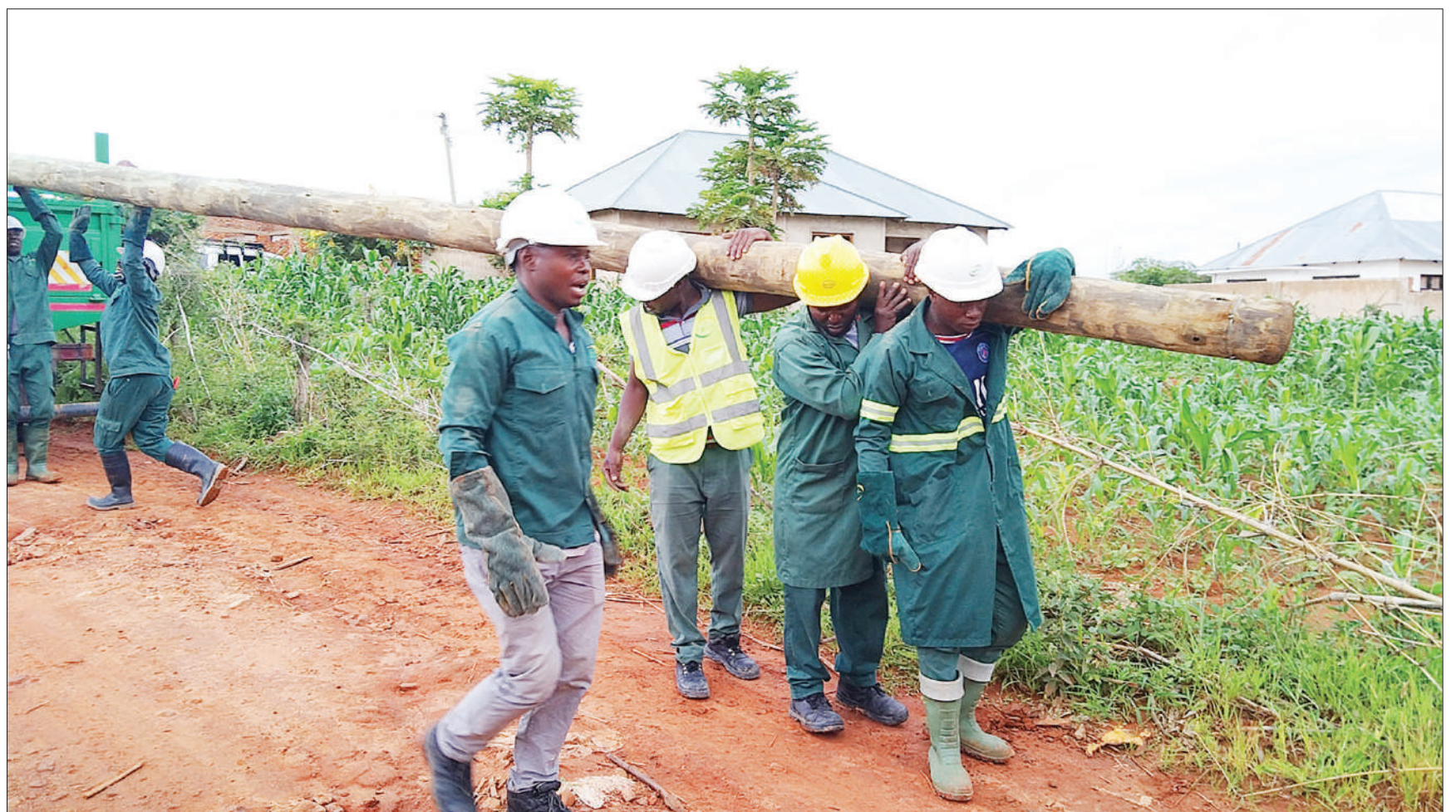
Tanzania Electric Supply Company (Tanesco) technicians pictured in the Kitwiro section of Iringa municipality yesterday moving to supply power to the over 2,170 people who have paid the required 27,000/- fee. Photo: Correspondent Francis Godwin
