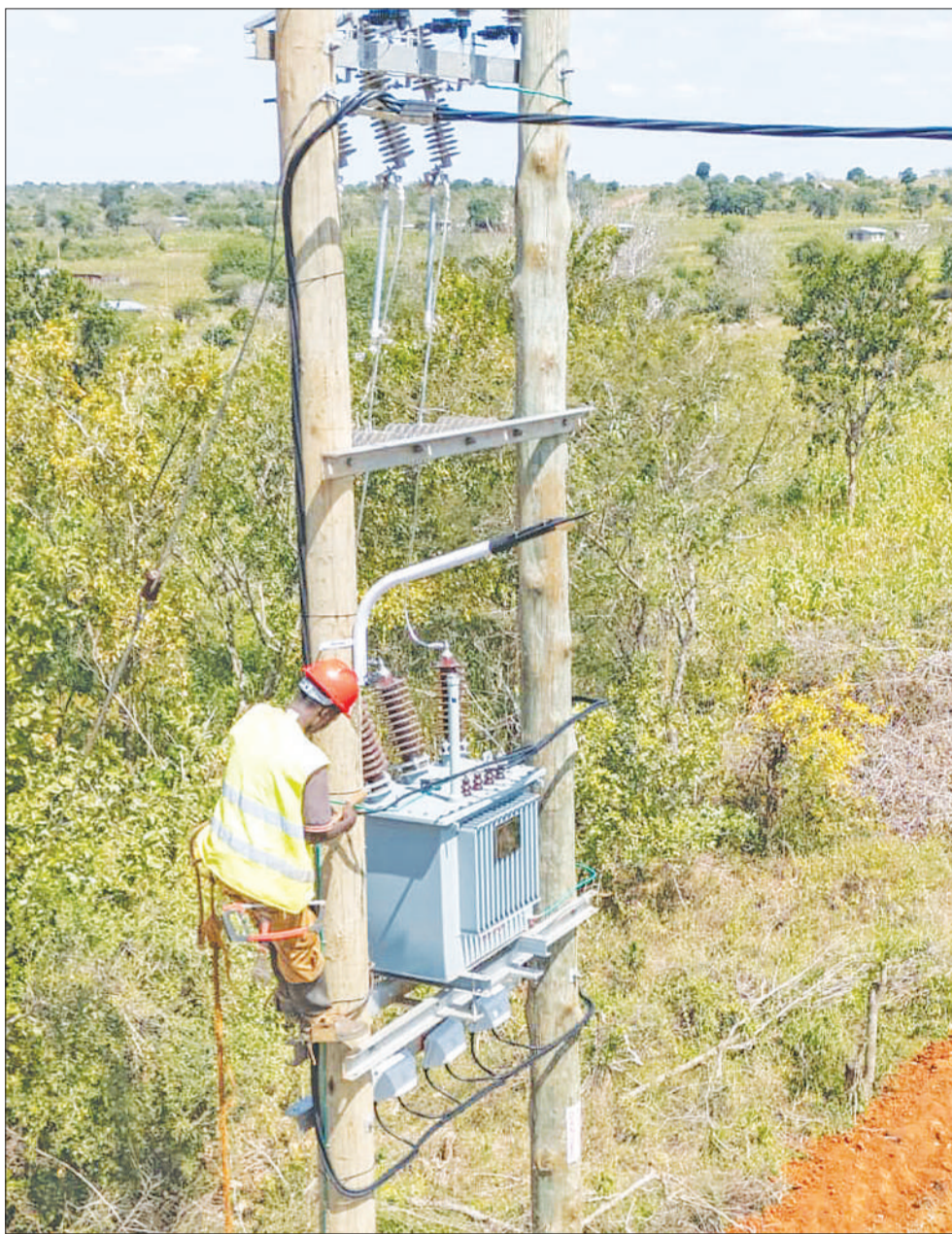
A technician with the Electrical Transmission Distribution Construction and Maintenance Company (ETDCO), a subsidiary of the Tanzania Electricity Supply Company Ltd (Tanesco), pictured yesterday installing a 132-kilovolt transformer as the implementation of the Tabora-Katavi electrification project continues. Story on Page 7. Photo: Guardian Correspondent
