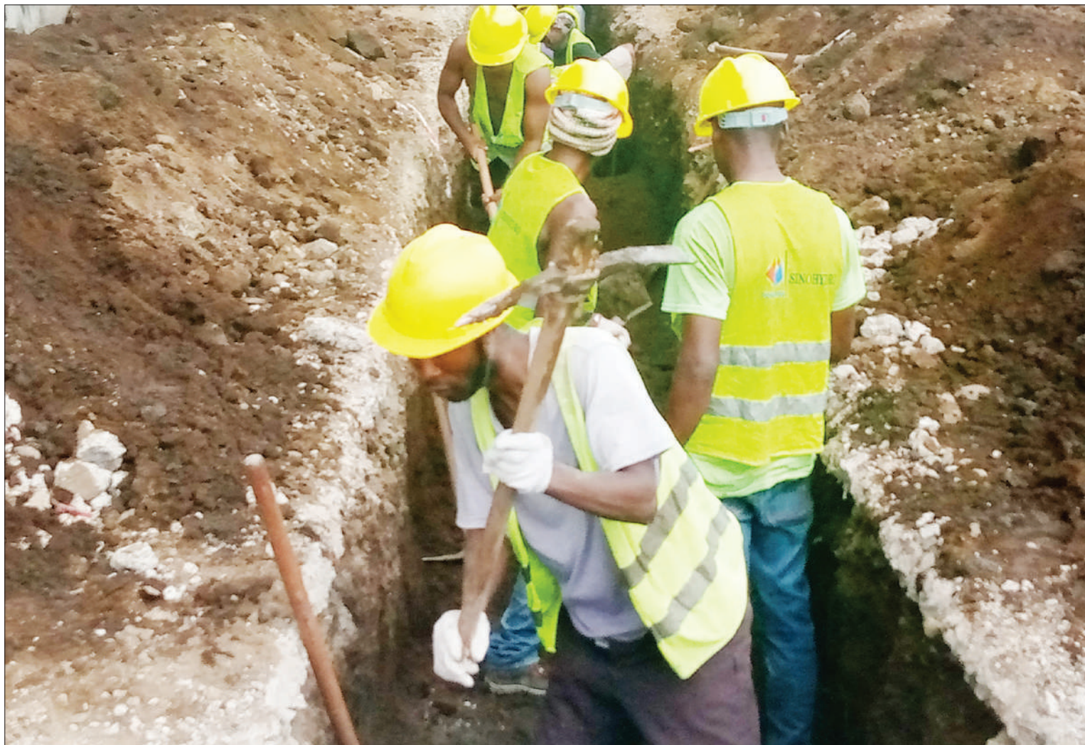
People engaged by China's Sinohydro Construction Company dig a sewage trench at a spot in the Esso section of Arusha city yesterday. Photo: Correspondent Daniel Sabuni
