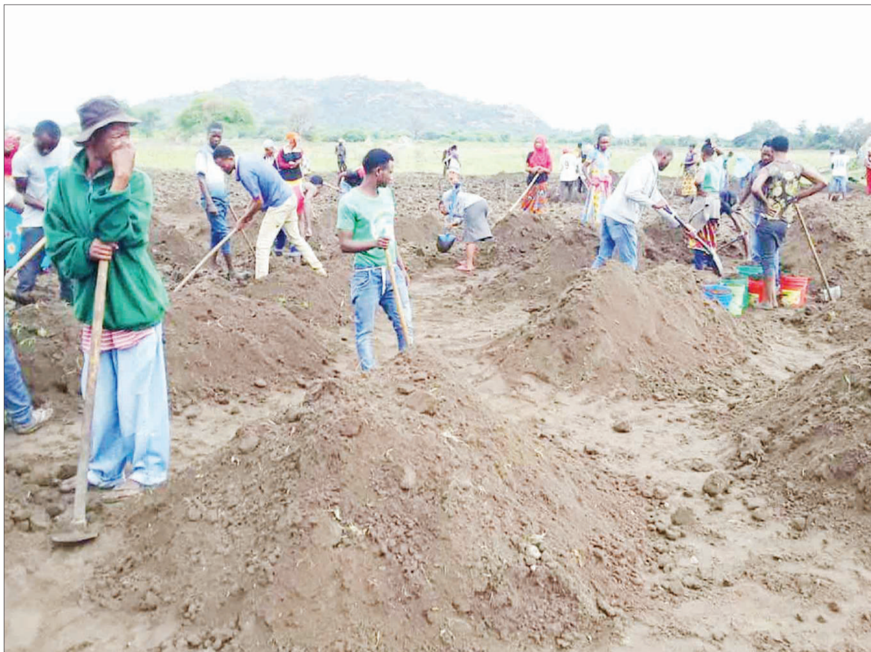
Residents of Mwada ward in Babati District, Manyara Region, pictured earlier this week preparing the site earmarked for the construction of a hospital. Photo: Guardian Correspondent
