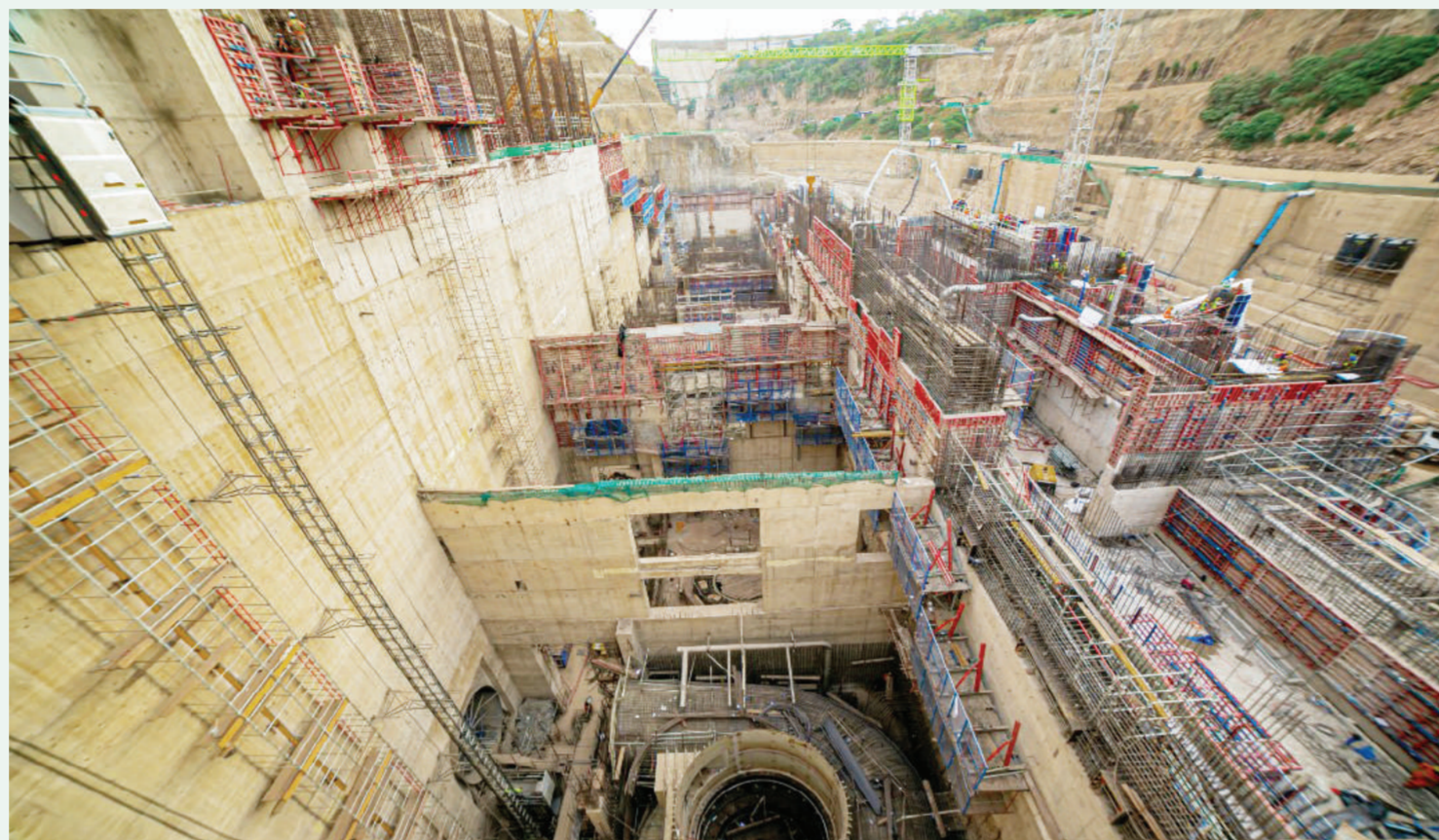
The special machinery operation block at the Julius Nyerere Hydropower Plant (JNHPP) project. Photo: Correspondent Valentine Oforo
