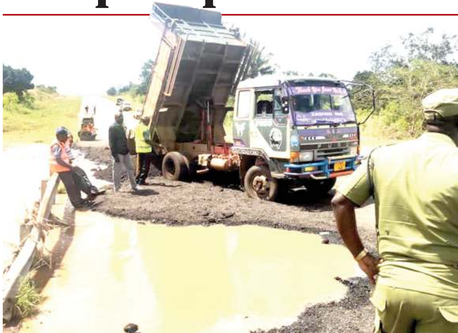
A Mandera (Coast Region) portion of the all-important highway linking Chalanze in Coast Region and Segera in Tanga Region - and leading all the way to Tanga, Moshi and Arusha and beyond - undergoes rehabilitation, as found at the weekend. It was so badly damaged by recent rains that it was temporarily closed to vehicular traffic for quite some time, leaving thousands of motorists and passengers stranded. Photo: Correspondent Boniface Gideon
