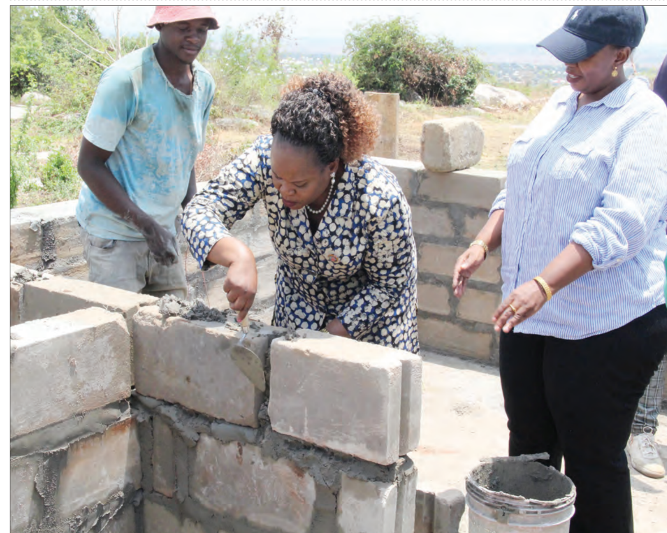
Shinyanga regional commissioner Christina Mndeme (C) temporarily turns 'bricklayer' on Thursday, lending a hand in construction work at the newly established Nyahanga Secondary School in Kahama municipality. Photo: Correspondent Marco Maduhu
