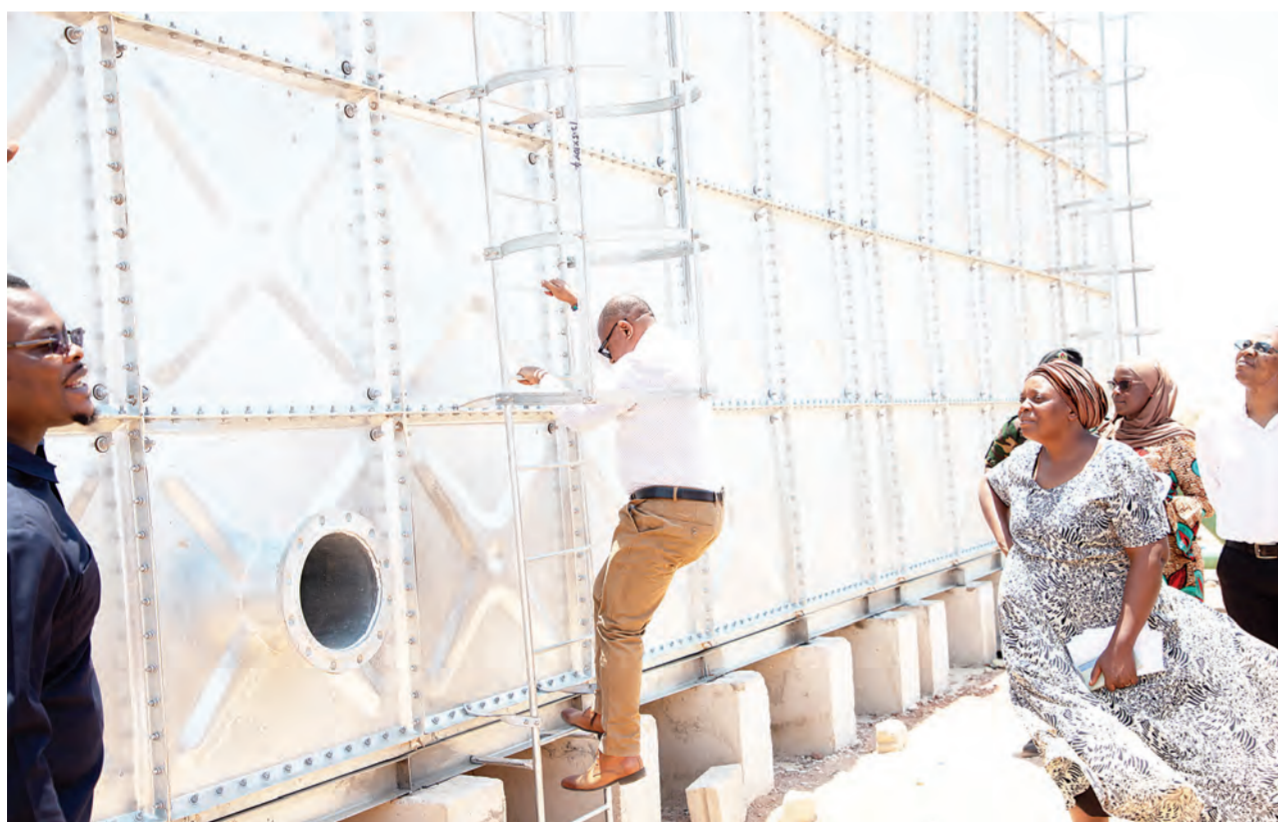
Dodoma district commissioner Jabir Shekimweri goes up the ladder yesterday to inspect a water tank while on an assessment tour of progress in the implementation of a project implemented by the Dodoma Urban Water Supply and Sanitation Authority in Nzuguni ward. Photo: Correspondent Peter Mkwavila
