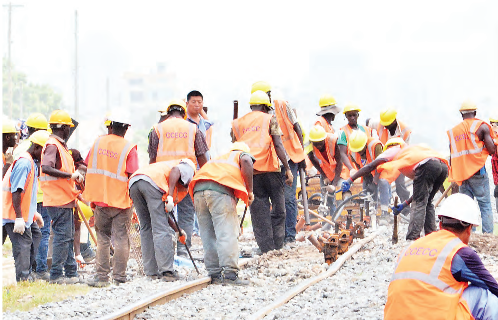
Rehabilitation of Central Railway in progress at Buguruni Chama in Dar es Salaam yesterday. Photo: Correspondent Miraji Msala
