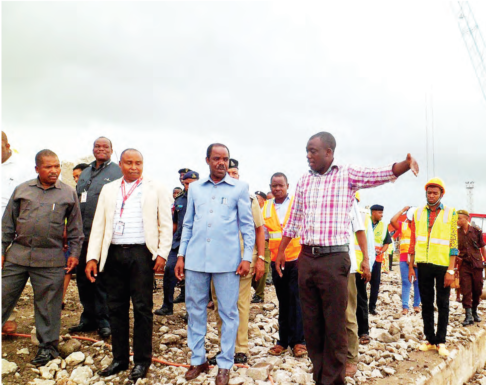
A Bico Engineering official (gesturing) updates Tanga regional commissioner Martin Shigella (to his right) yesterday on the deepening of Tanga Port, work meant to make the facility more efficient and able to handle larger cargo ships than is now the case. Photo: Correspondent Boniface Gideon
