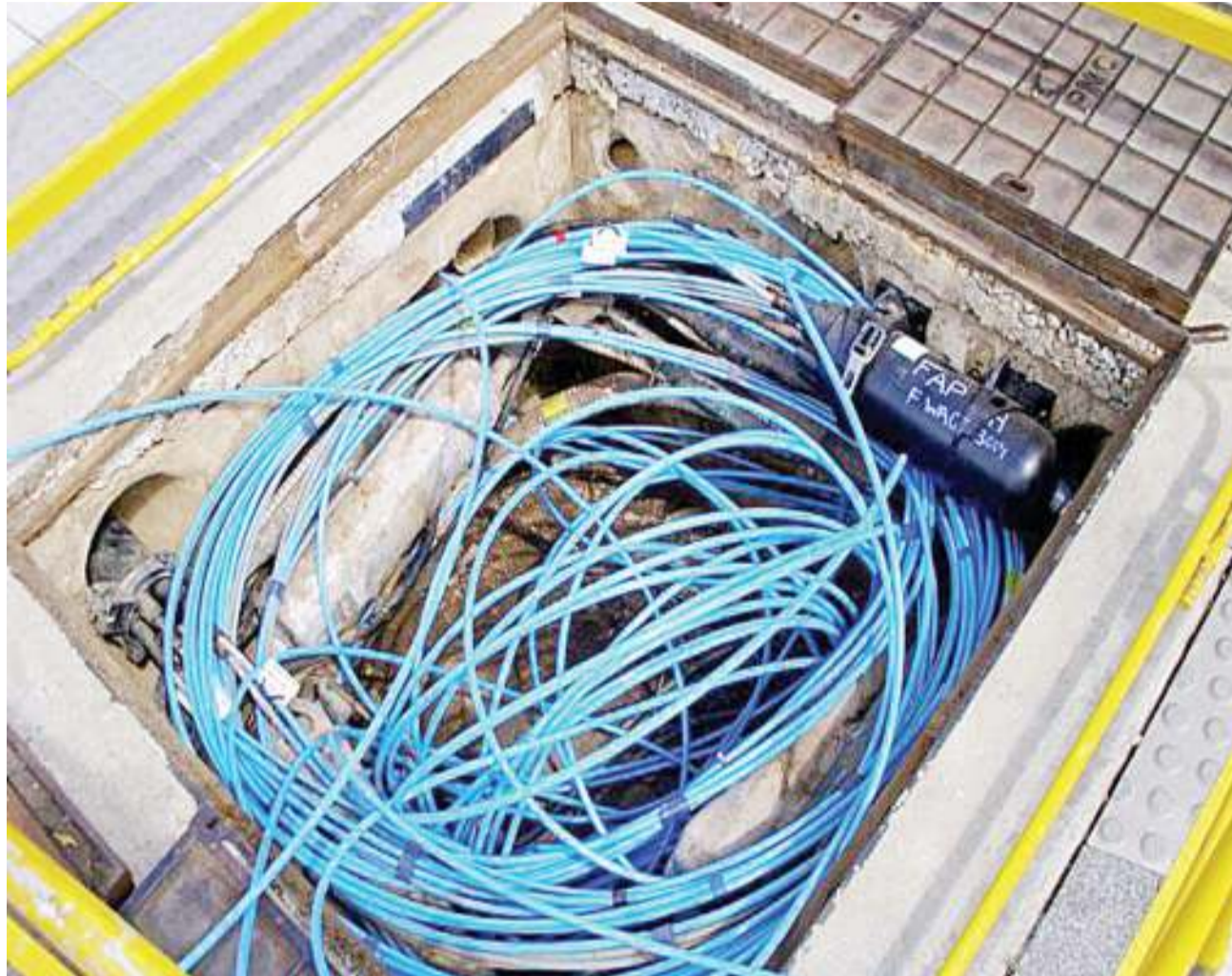
An open underground fibre optic cable vault in Nairobi.
