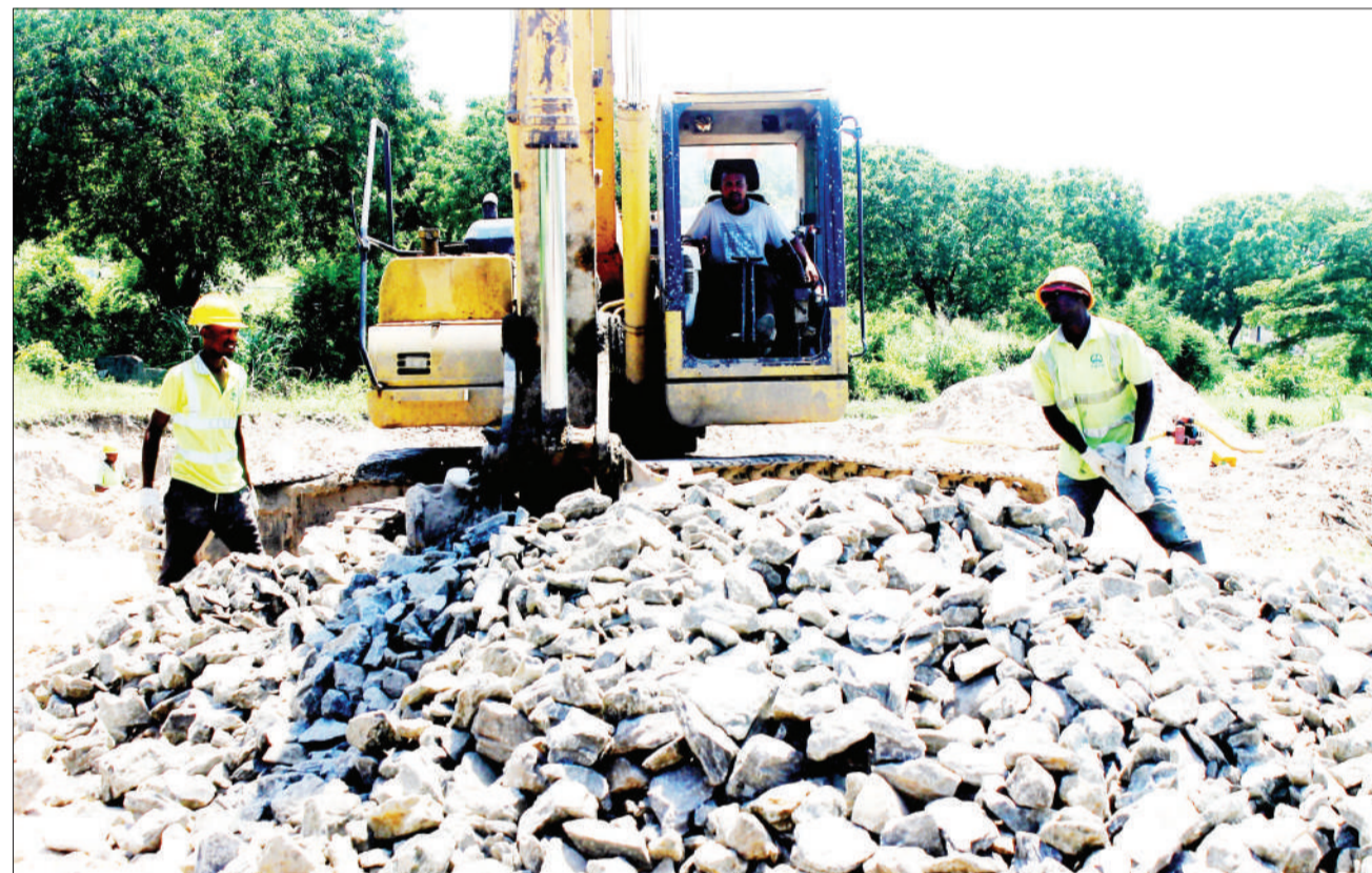
Masons systematically arrange stones yesterday in an effort to protect the Kigamboni segment of Dar es Salaam's Indian Ocean shore from erosion by raging sea waves. The operation has gone on for years, with qualified success. Photo: Correspondent Jumanne Juma
