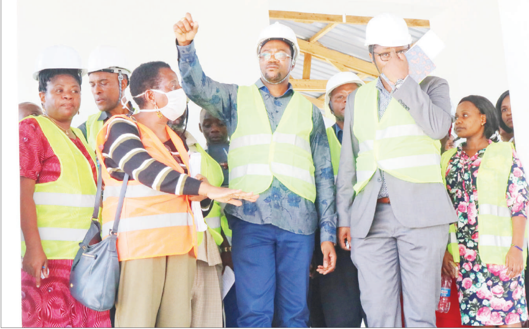
Y&P Architects consultant Anna Shayo (2nd-L), who is supervising the construction of the Tanzania Fishing Research Institute laboratory in Dar es Salaam, briefs Livestock and Fisheries minister Luhaga Mpina (C). The latter toured the site of the project at Kunduchi yesterday. Photo: Guardian Correspondent
