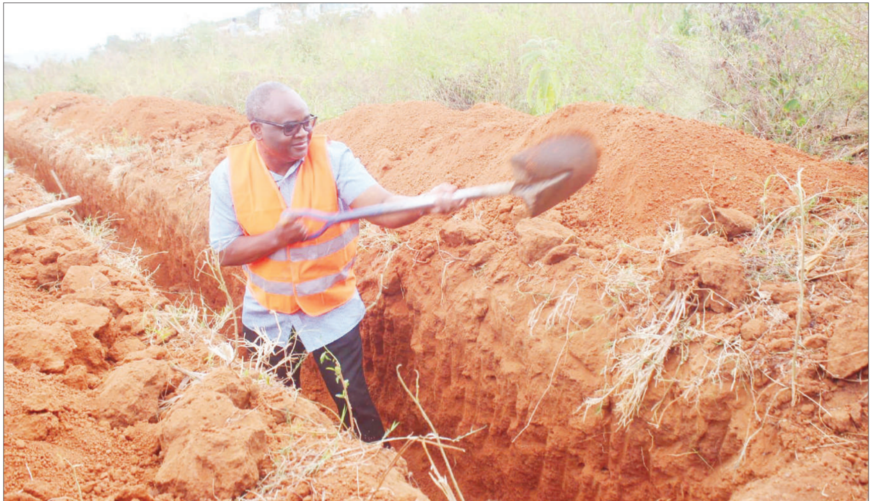
Water ministry permanent secretary Prof Kitila Mkumbo takes part in the digging of a tunnel in which to lay a pipe to supply water to Chato airport in Geita Region, as captured yesterday. Photo: Correspondent Mohamed Saif
