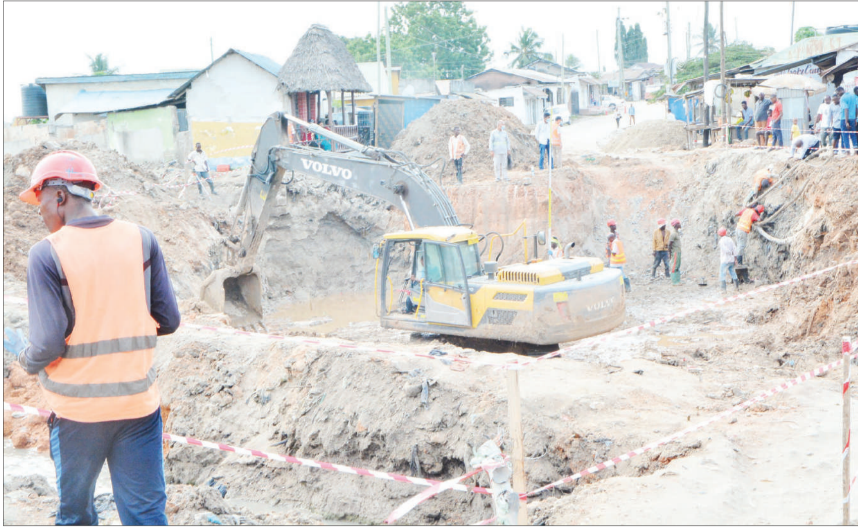
Expansion of Dar es Salaam's River Ng'ombe gets under way at the Kwa Mtogole section in Kinondoni District yesterday. The idea is to ensure that the river no longer bursts its banks, with water invading residential and other buildings. Photo: Correspondent Miraji Msala
