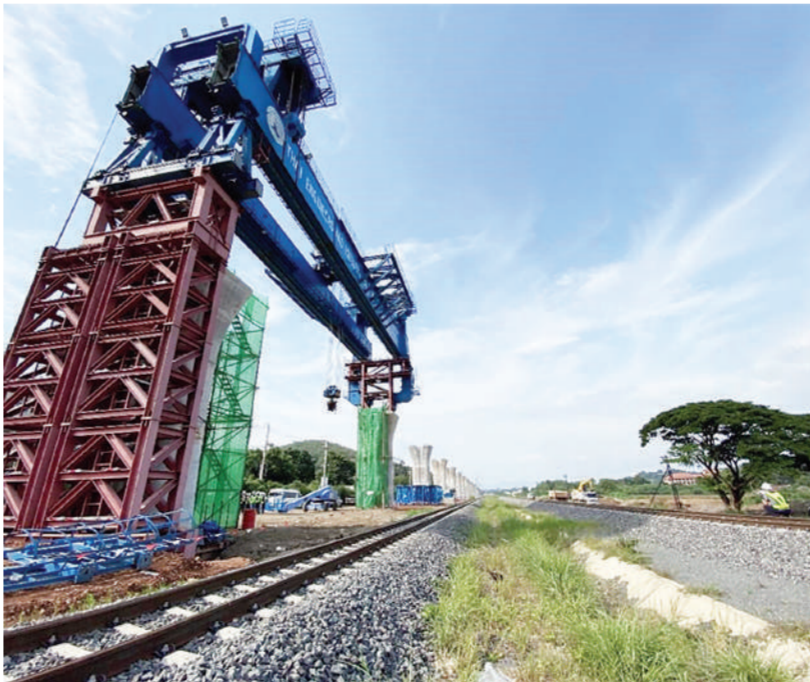
Photo shows a construction site of the first phase project of the China-Thailand railway in Nakhon Ratchasima province, Thailand. File photo
