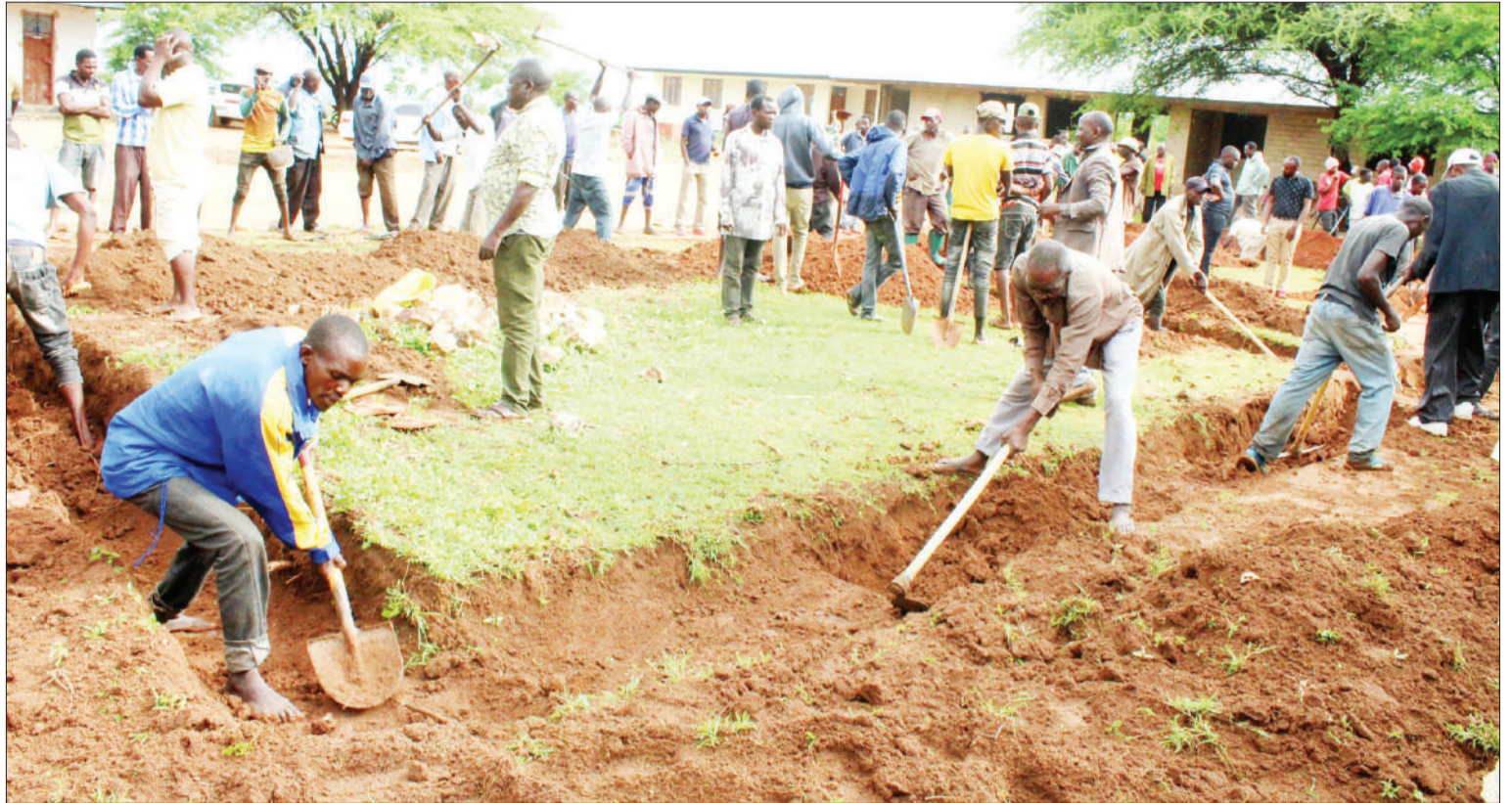
Kolandoto ward residents in Shinyanga municipality digging two classrooms foundation at Kolandoto secondary school following the shortage facing the school. Photo: Correspondent Marco Maduhu
