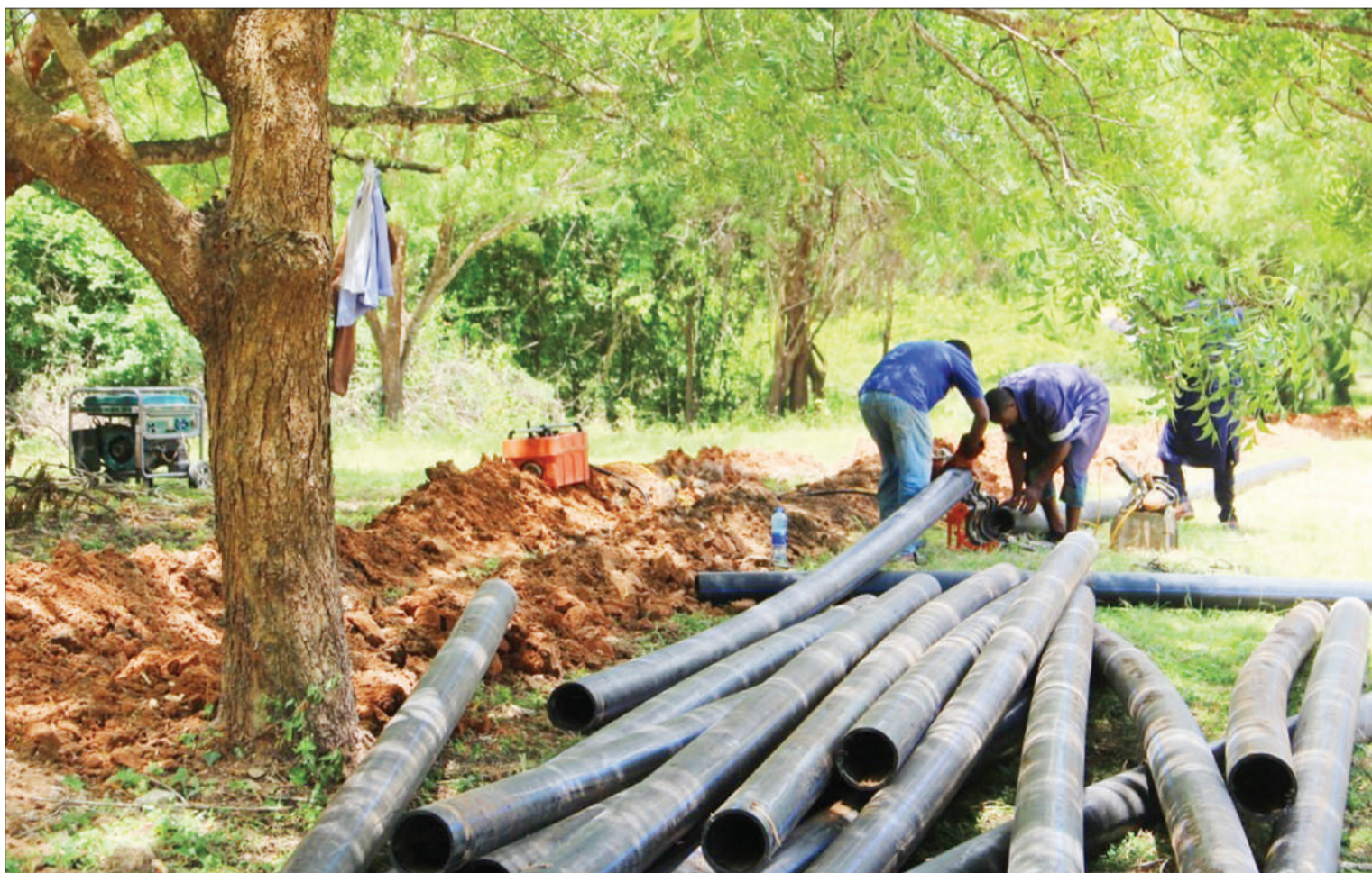
Dar es Salaam Water and Sanitation Authority technicians laying and joining water pipes at the Ardhi University's hostel to improve the services at the area yesterday. Photo: Guardian Correspondent
