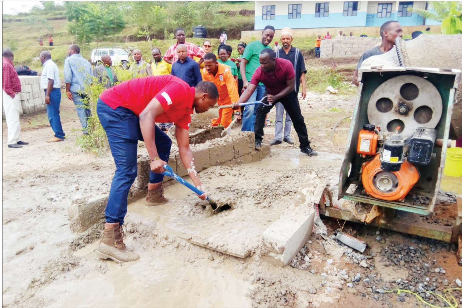
Arusha District Commissioner Kenan Kihongos participates in classrooms construction at Muivaro secondary school yesterday. Photo: Correspondent Tmaini Mafie
