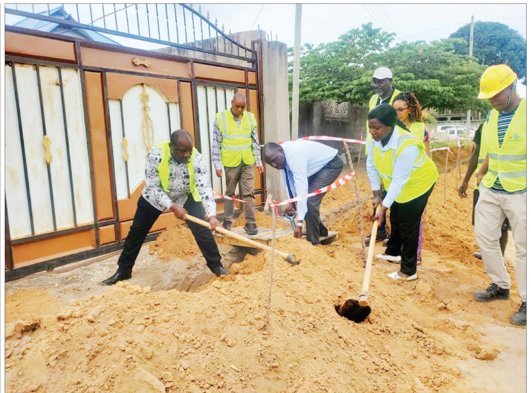
Kinondoni District Commissioner Daniel Chongolo (L) takes part to dig a trench to lay a pipe as part of the Dar es Salaam Water and Sanitation Authority strategy to improve water services at Makongo suburb. Photo: Guardian Correspondent
