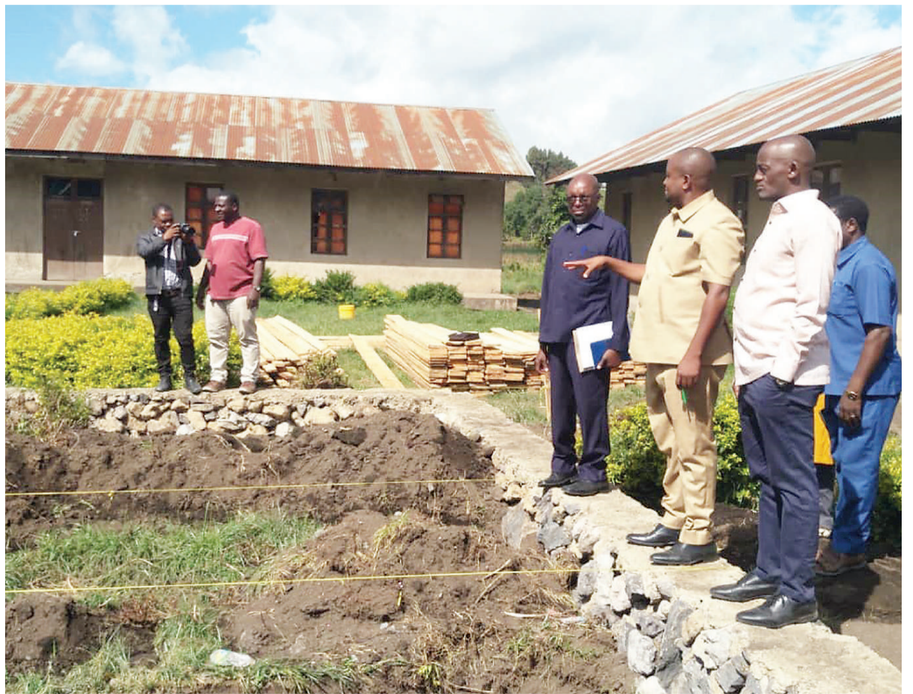
Representatives of the Mbeya District Commissioner's Office have a first-hand account of progress in the construction of classrooms at Iwalanje Secondary School at the weekend. Photo: Correspondent Nebart Msokwa
