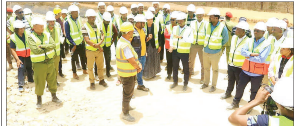
Minister of State, President Office, Union and Environmental, Selemani Jafo during his special tour of the ongoing Julius Nyerere Hydropower Station (JNHPP) hydroelectric dam construction project in Rufiji River. The Minister paid a special visit of the country's mega- power project to inspect the state of environmental. Photo: Correspondent Valentine Oforo
