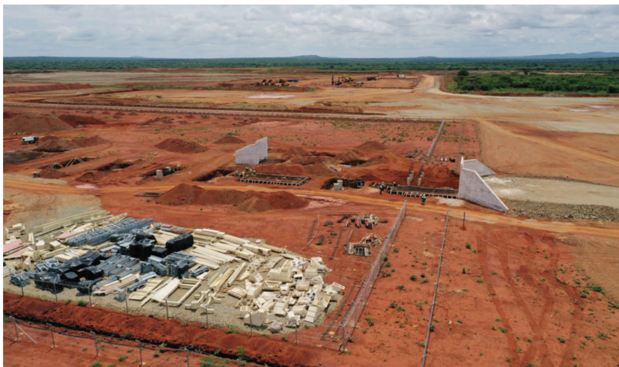
Singida Gold project's process plant site PHOTO/SHANTA
