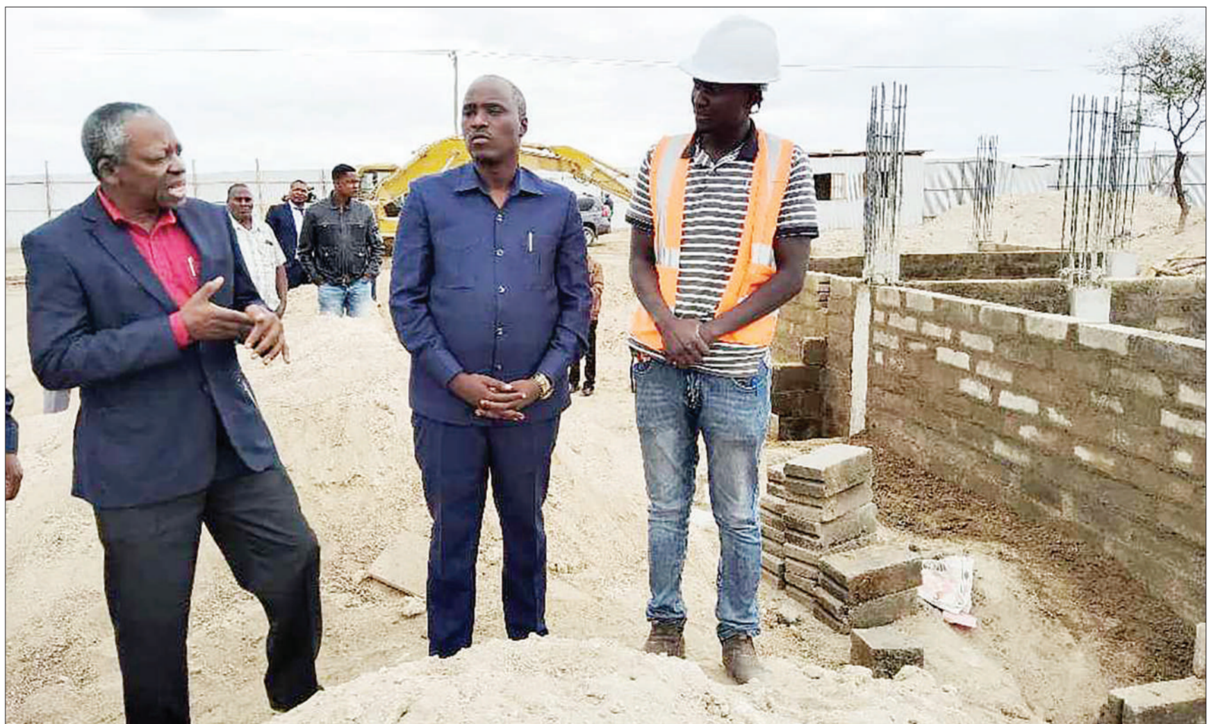
Manyara Regional Commissioner Charles Makongoro Nyerere (L) explains about the progress reached in the construction of the Tanzanite mineral market building, in the small town of Mirerani, Simanjiro District to the Minister of Mines, Dotto Biteko (C), after his inspection. The government offered 1.5 billion/- for the construction of the market. Photo: Correspondent Gift Thadey
