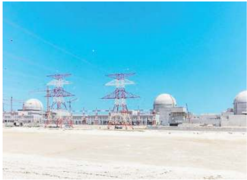
This handout photo released by the Emirates Nuclear Energy Corporation (ENEC) on June 1, 2017 shows part of the Barakah nuclear power plant under construction near al-Hamra, west of Abu Dhabi, in May 2017. (AFP)
