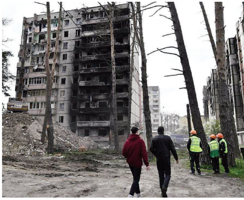
Local residents walk past a heavily damaged residential building as workers dismantle it in the town of Irpin, on April 19, 2023. AFP
