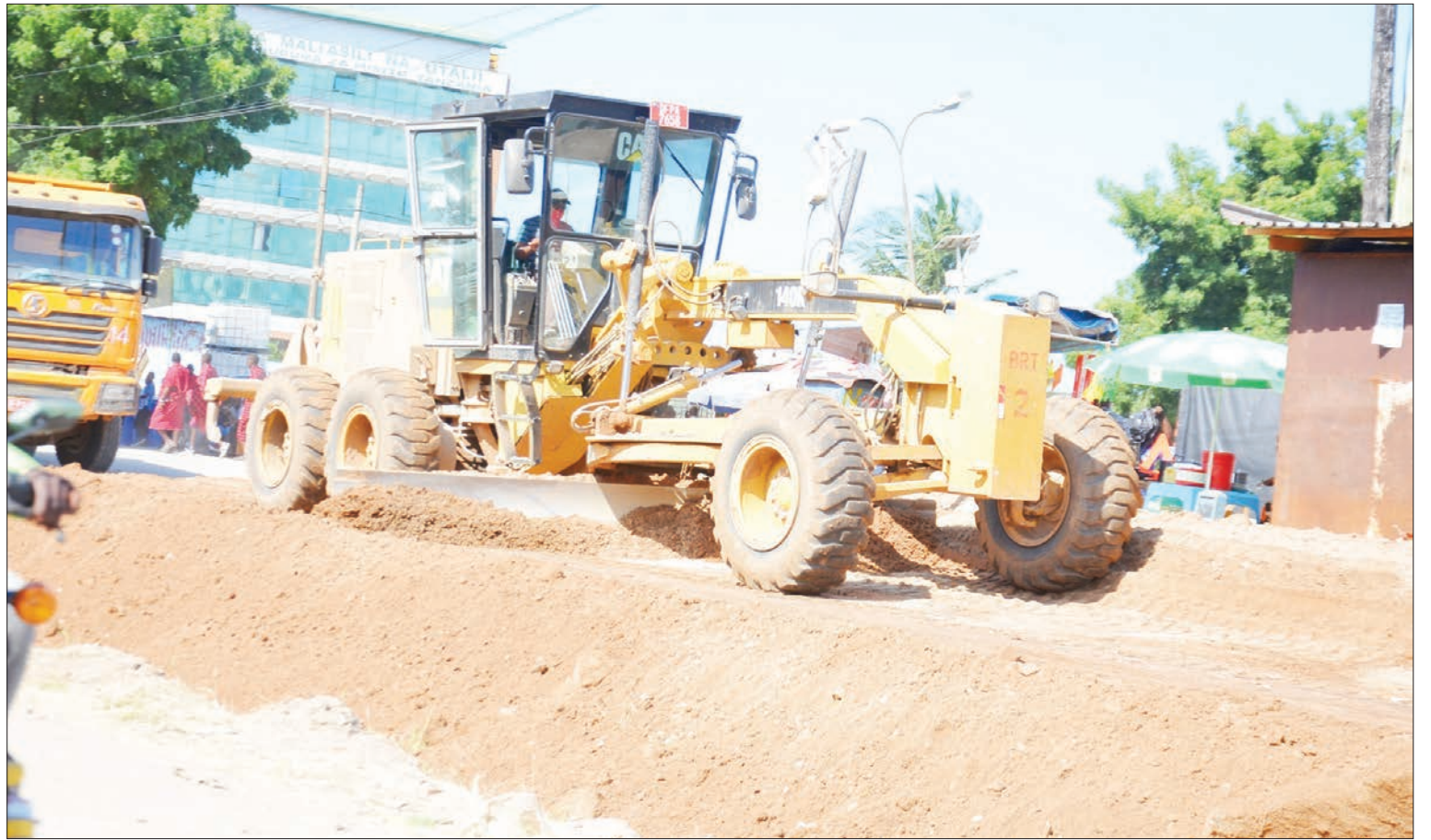
Construction of a flyover at the junction of Nyerere/Kawawa road in Dar es Salaam. Photo: Correspondent Jumanne Juma
