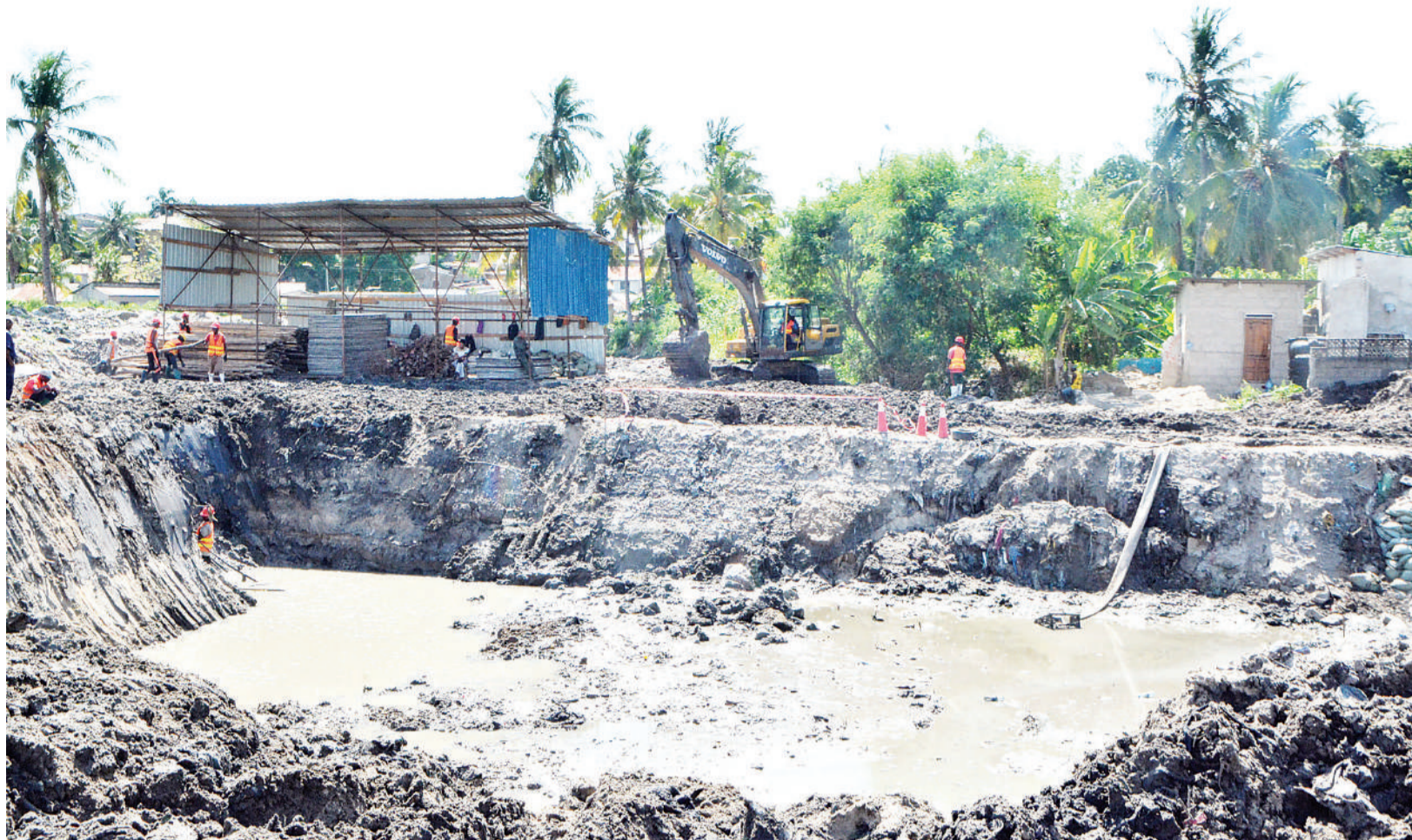
Construction of a bridge to link Dar es Salaam's Magomeni Kwa Harubu and Mwananyamala suburbs well under way yesterday. Photo: Correspondent Miraji Msala
