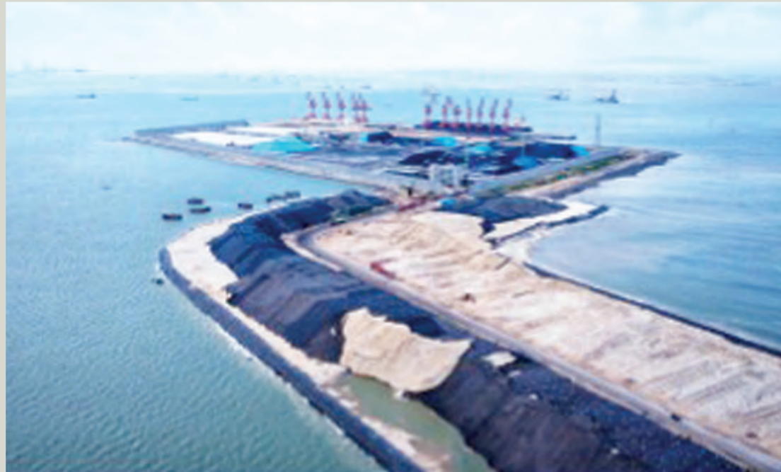
Photo taken in June 2021 shows an expansion project for the east channel of Qinzhou Port, south China's Guangxi Zhuang autonomous region. Upon completion, the port will have a two-way route that stretches 23.23 kilometers and is navigable to 100,000-ton containerships. File photo
