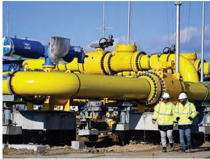
employees walk at the construction site of a gas metering station, part of the pipeline link between Bulgaria and Greece near the village of the
