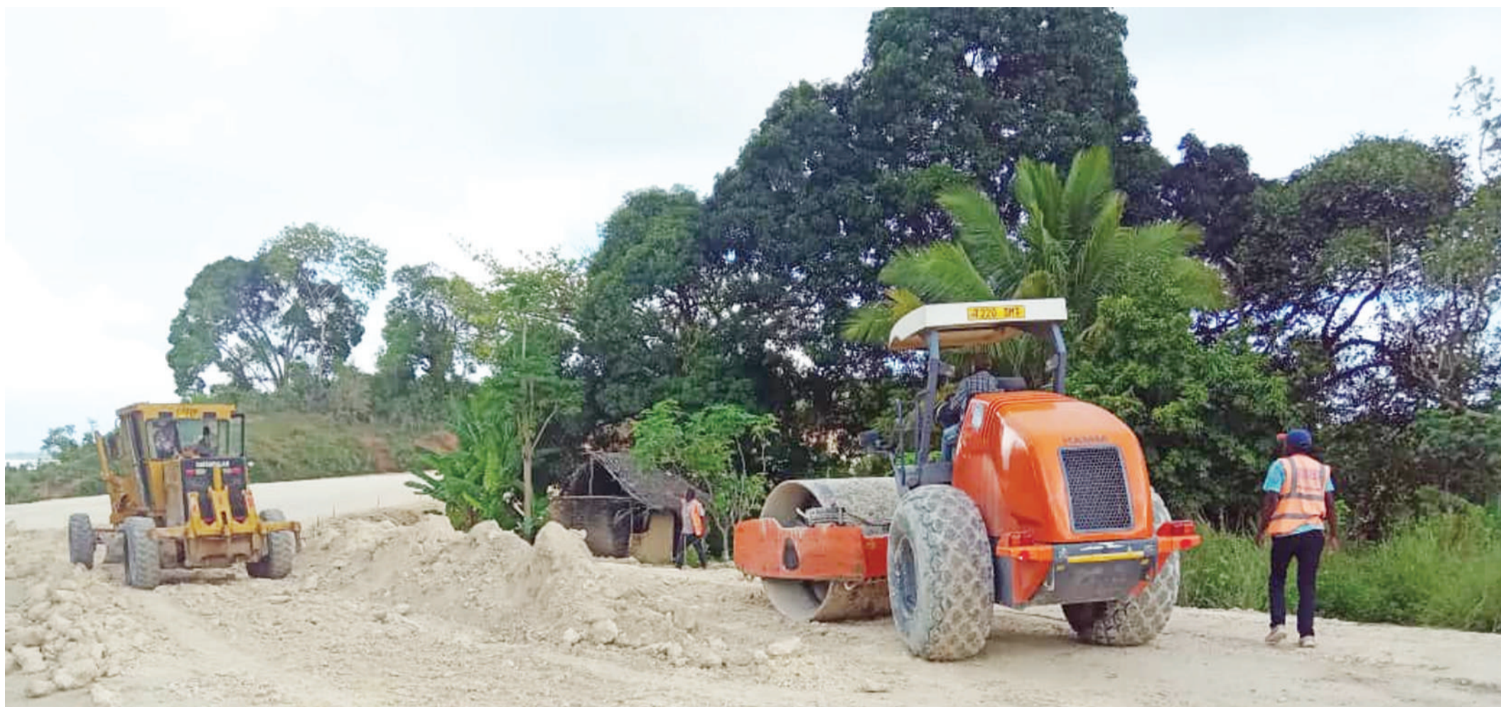
Construction of Chakekake-Wete road in North Pemba Region in progress, as found last week. Photo: Guardian correspondent
