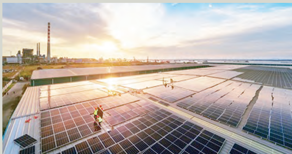
Solar panels are being installed in an industrial base in Ma'anshan, east China's Anhui province, November, 2021. File photo
