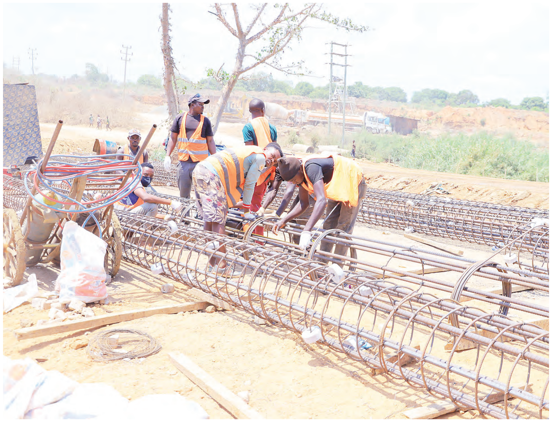
Technicians with the company building the 53.2-km Ruangwa-Nanganga road to tarmac level as well as Lukuledi Bridge – in Lindi Region – busy at work on the strategic bridge at the weekend. Photo courtesy of Works ministry
