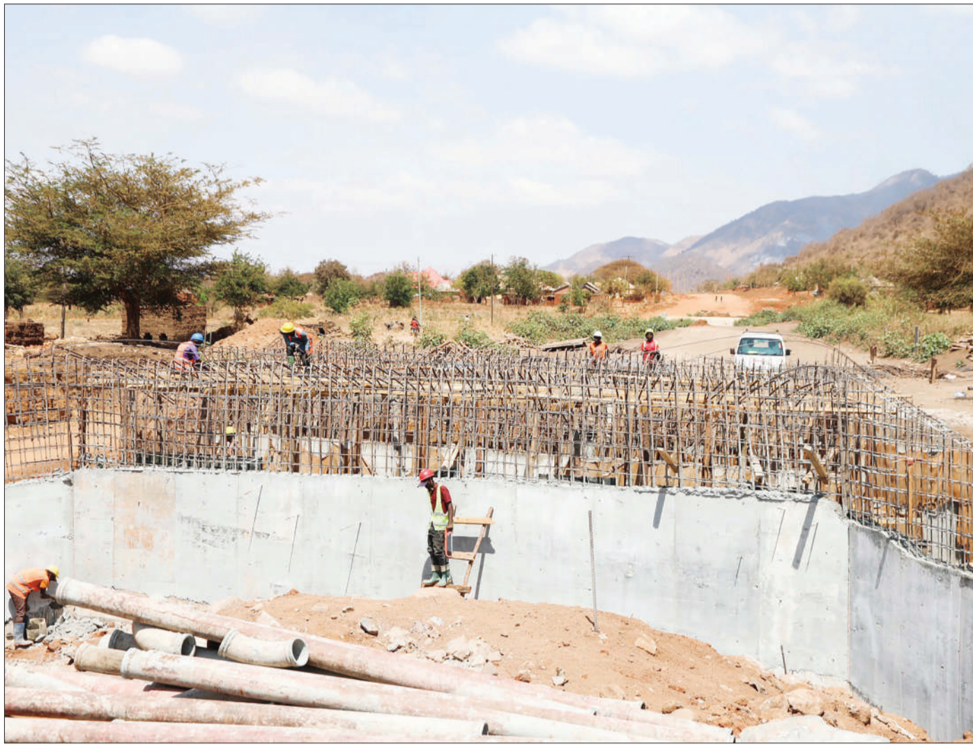
Construction a bridge in Mpwapwa District in progress, as found yesterday, this being part of the government's strategy to improve surface transport in Dodoma Region. Photo: Guardian Correspondent
