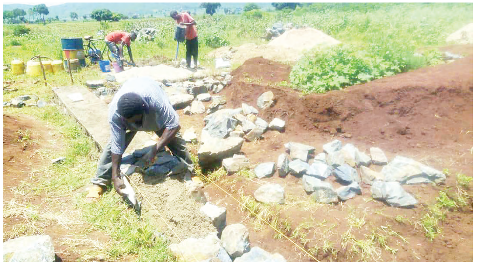
Preparations for the construction of Seka Secondary School under way in Nyamrandirira ward in Musoma Rural constituency earlier this week, with both the government and residents of the area contributing to the implementation of the project. Photo: Guardian Correspondent
