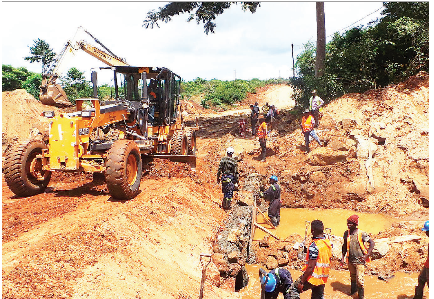
Construction of a side road meant to pave the way for major rehabilitation of a strategic bridge at Kiyegeya in Morogoro Region recently swept away by floodwaters in progress. The bridge lies along the Morogoro-Dodoma highway. Photo: Guardian Correspondent
