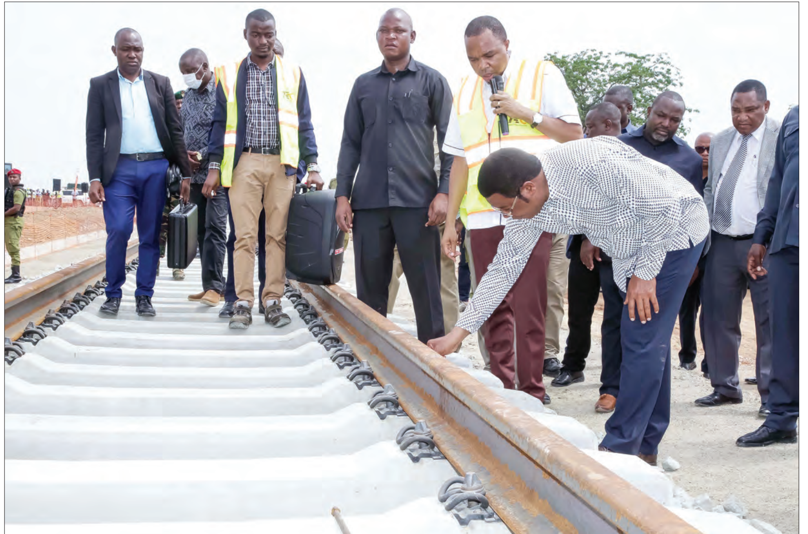
Prime Minister Kassim Majaliwa has a first-hand account yesterday of the ongoing implementation of the second phase – Morogoro to Makutupura in Dodoma Region – of the standard gauge railway project. This was along the Ihumwa-Igandu stretch. Photo: PMO
