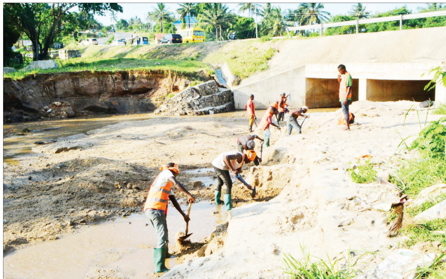
Efforts to remove sand from Dar es Salaam's near-choked Tegeta River and expedite the flow of water under the strategic Goba Bridge under way along Madale Road at the weekend. Photo: Correspondent Miraji Msala
