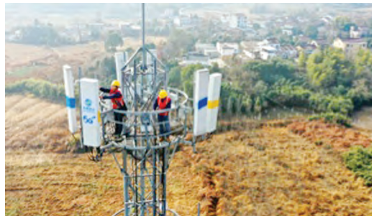
Photo taken on Dec. 13, 2021 shows network maintenance workers testing and adjusting 5G base station antennas at Shuicun village, Zhongming township, Yi'an district, Tongling city, east China's Anhui province. File photo
