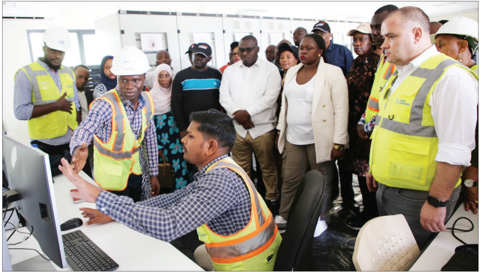
Tanzania Railway Corporation Engineer Kusyama Lameck briefs Members of the Parliamentary Standing Committee on Public Capital Investment (PIC) regarding the high-speed rail (SGR) cooling plants at the Pugu station in Dar es Salaam yesterday. Photo: Parliament
