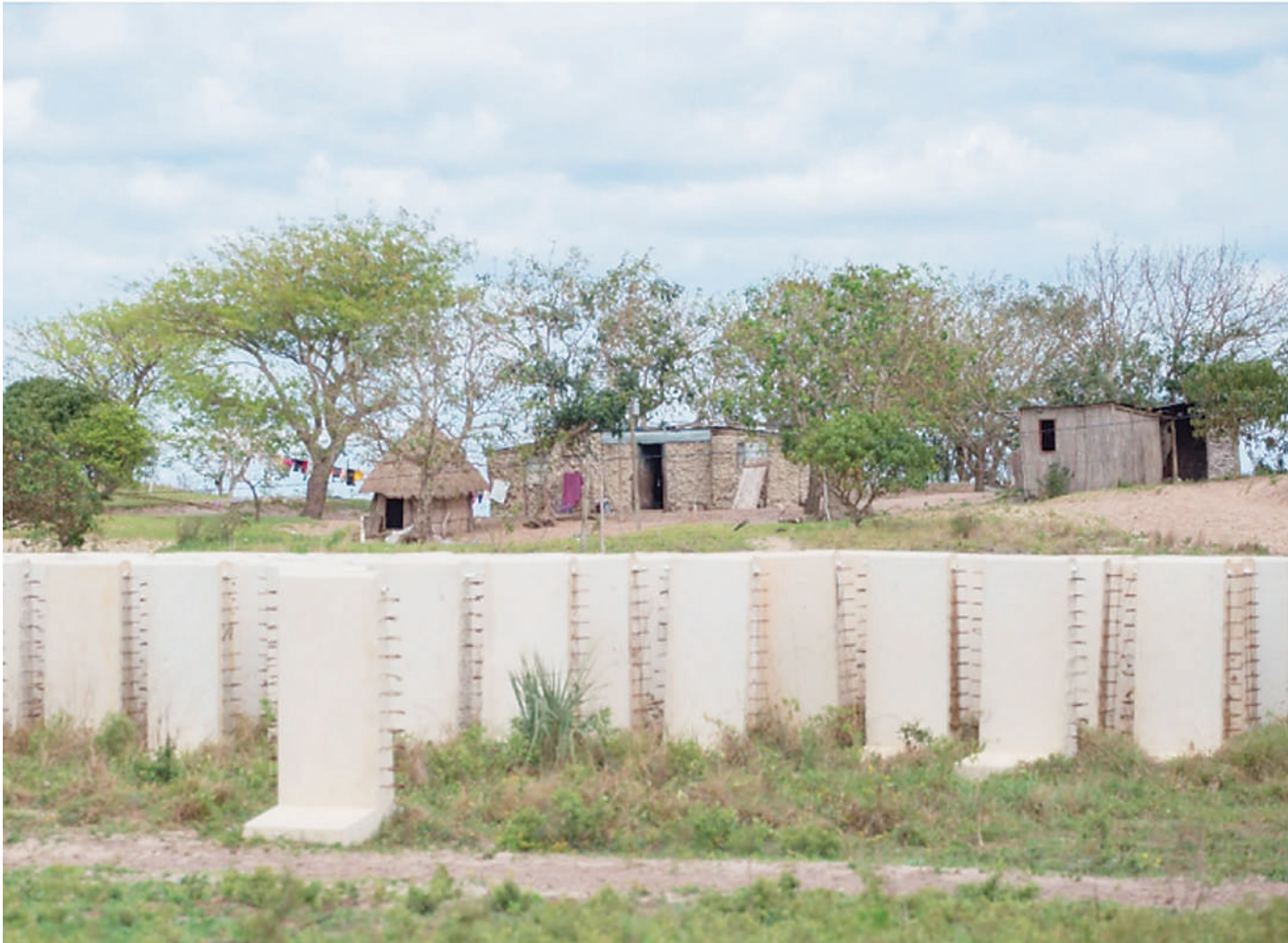
Concrete barriers that are not yet operational but are intended to separate Manguzi and Mozambique as an anti-crime barrier. By 2020, only 166m of the wall had been constructed, even though R48m was paid to the contractor. The amount should have covered the cost of installing 3km of border wall. The SIU is investigating. (Photo: Supplied)
