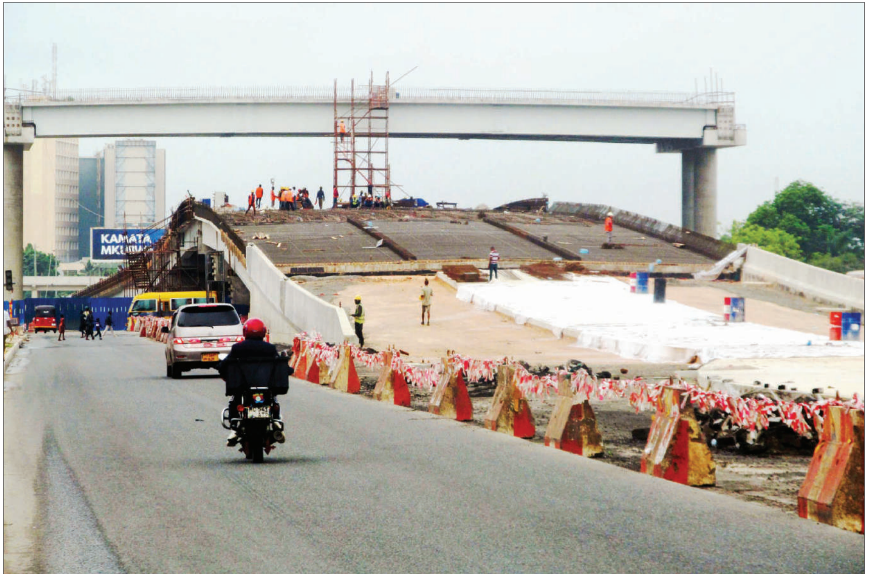
Part of the interchange bridge which is under construction at the junction of Ubungo, Mandela Express Highway and Sam Nujoma Road in Dar es Salaam as captured yesterday by our roving photographer. Photo: Correspondent Sabato Kasika
