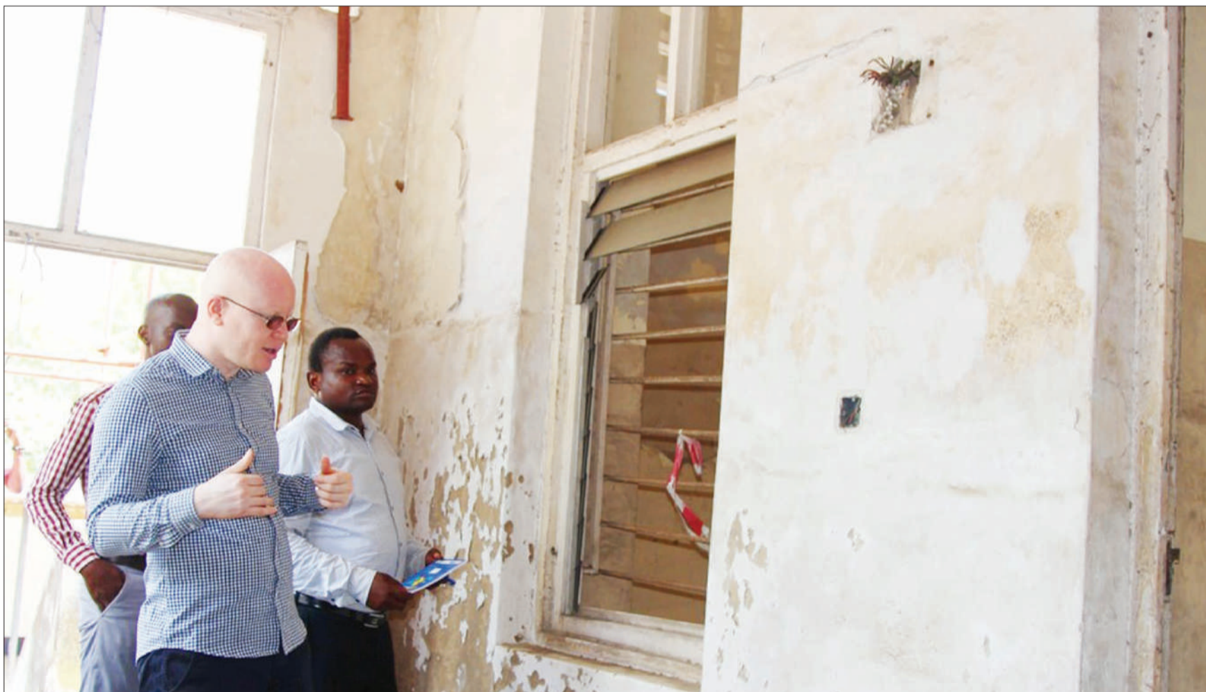
Information, Culture, Arts and Sports deputy Permanent Secretary Dr Ally Possi (R) inspects former headquarters of the committee of Liberation of the African Continent which is under rehabilitation aimed to protect African history in Dar es Salaam over the weekend. With him is cultural officer Christopher Mhongo. Photo: Information Services
