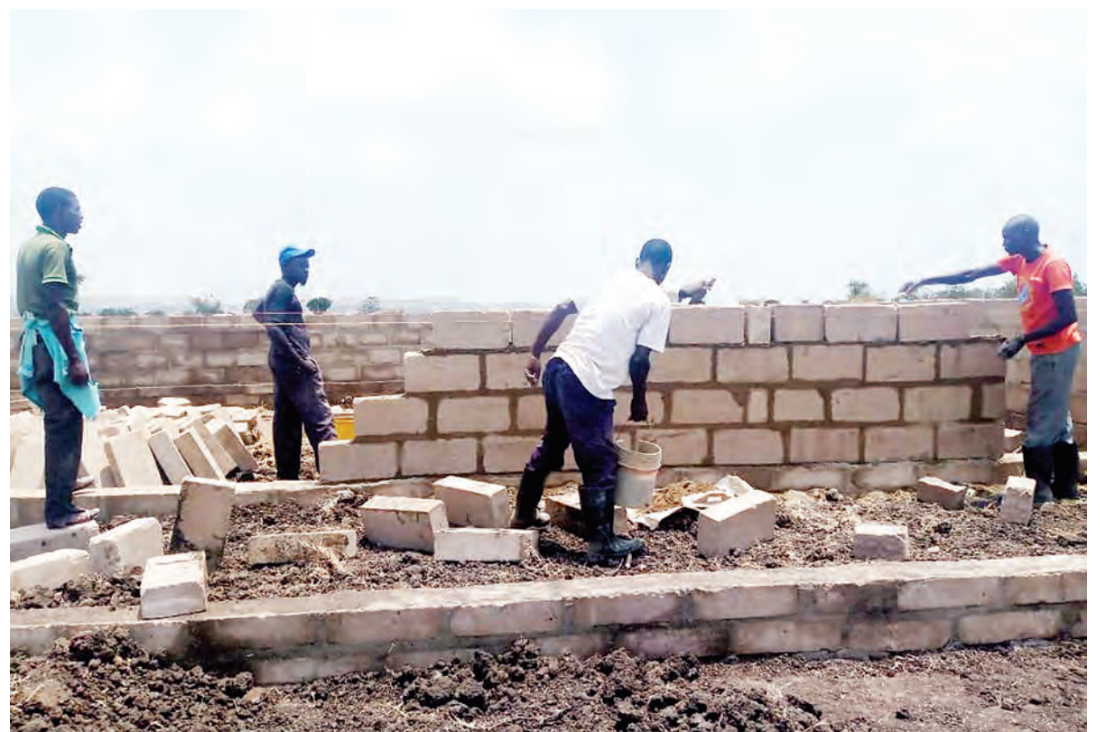
Construction of a building in progress at a newly established nursery school at Gomora in Musanja village, Musoma District, earlier this week. Photo: Guardian Correspondent
