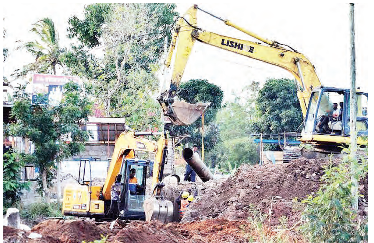
Installation of water pipes between Dar es Salaam's Goba and Madale suburbs well under way, as found yesterday. Photo: Correspondent Miraji Msala
