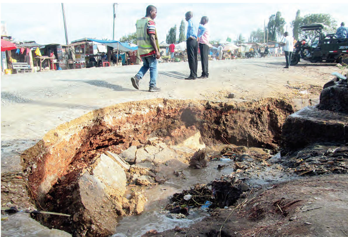
This is graphic evidence of the damage earlier this week's rains did to a section of a road under construction to tarmac level in Dar es Salaam's Mabibo suburb, as captured yesterday. Photo: Correspondent Sabato Kasika
