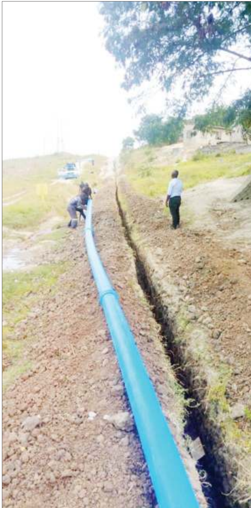
Dar es Salaam Water and Sewage Authority workers lay pipes for relaying water to the city's Kimara Golani suburb, as found yesterday. Photo: Guardian Correspondent
