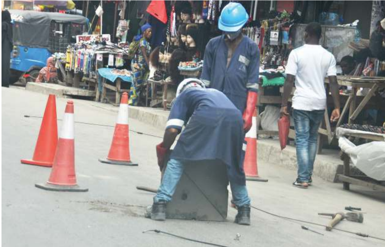
Technicians unblocking wastewater along Uhuru Road at Kariakoo area in Dar es Salaam yesterday. Photo: John Badi
