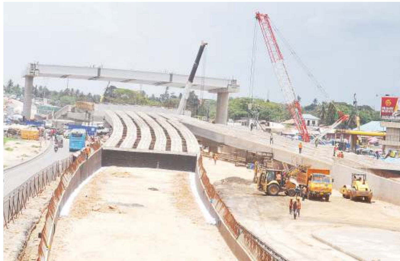
A view of a section of ongoing construction of Ubungo Interchange at the junction of Morogoro Road and Mandela Expressway as captured by our roving photographer in Dar es Salaam yesterday. Photo: John Badi
