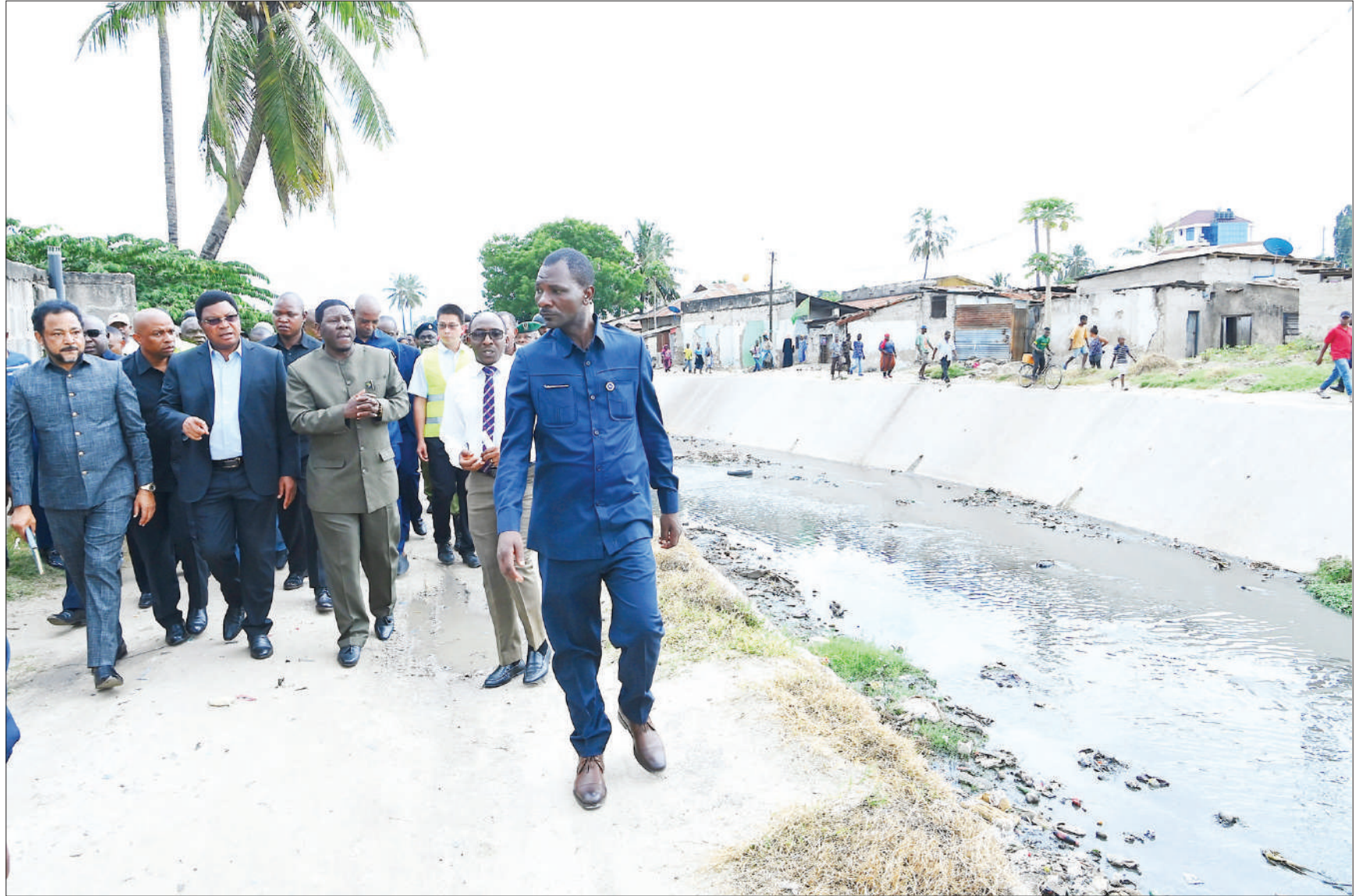
Prime Minister Kassim Majaliwa pictured in Dar es Salaam yesterday having a first-hand account of the construction of a canal designed to tame the Tandale-kwa-Mtogole stretch of River Ng'ombe in Kinondoni District, his delegation including Kinondoni Municipal mayor Songoro Mnyonge, Kinondoni legislator Abbas Tarimba, and Kinondoni district commissioner Godwin Gondwe. Photo: PMO
