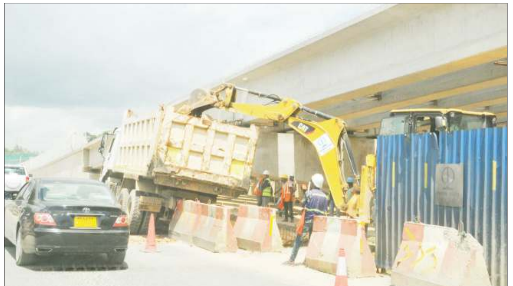
The appearance of a section of Dar es Salaam's Ubungo Interchange - at the Morogoro Road/Mandela Road/Sam Nujoma Road intersection - which is still under construction. This scene was captured yesterday. Photo: John Badi
