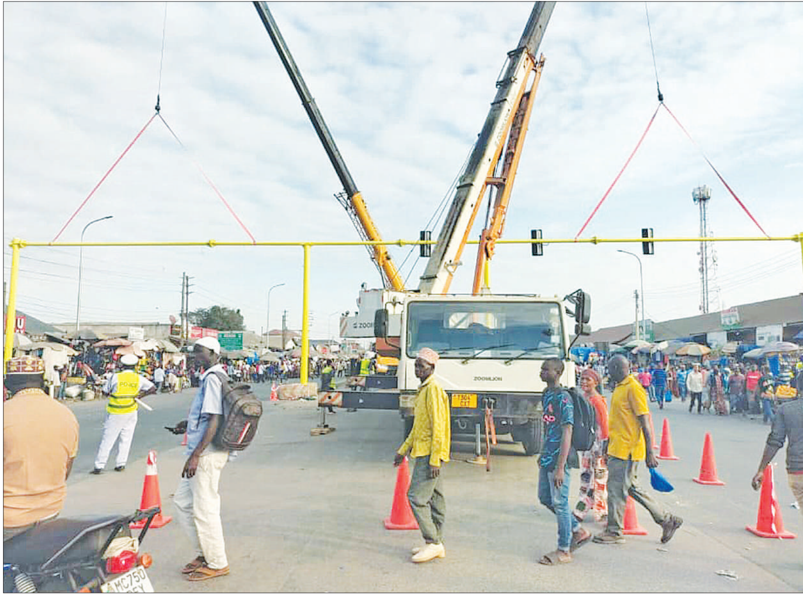
Construction of street lighting infrastructure in progress yesterday at a Kilwa Road section of Dar es Salaam's Bus Rapid Transit project site. Photo: Guardian Correspondent
