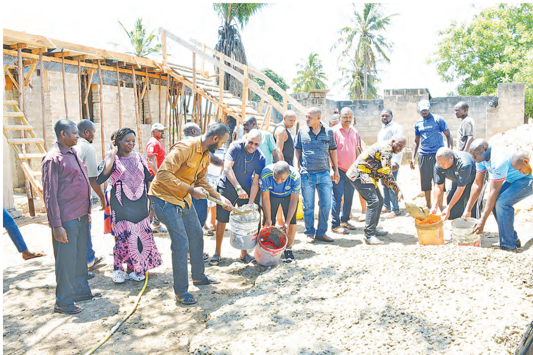
Residents of Goba in Kinondoni District, Dar es Salaam Region, pictured yesterday taking part in the construction of a police station building in the suburb on a self-help basis. It was reported that they have so far contributed 12m/- towards the implementation of the project. Photo: Correspondent Miraji Msala
